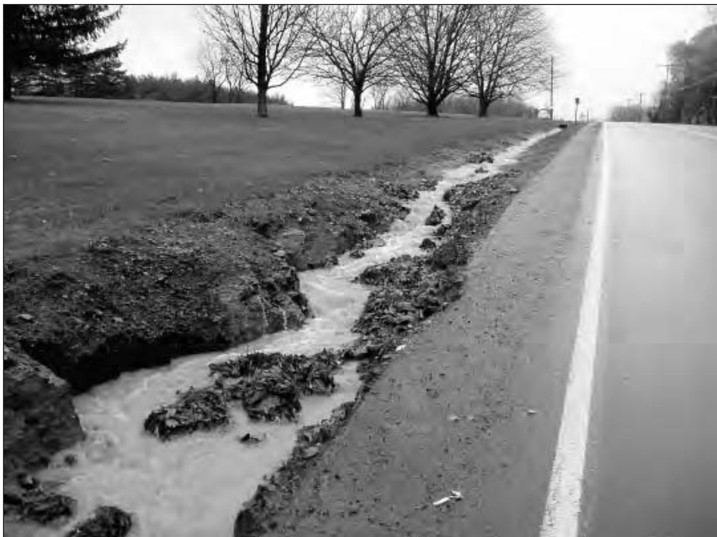
A turbid discharge from a residential subdivision under construction that flowed into a Class C trout stream.
