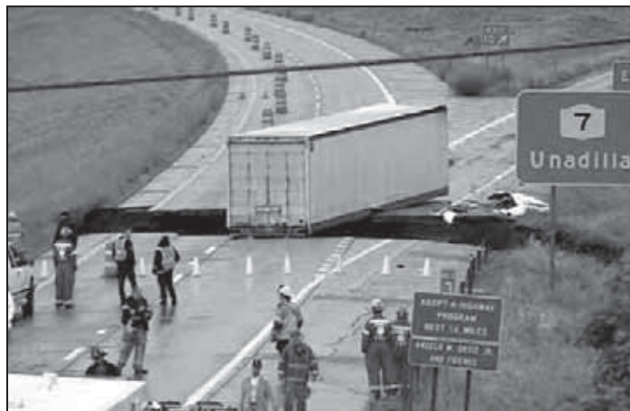
Emergency personnel respond to the I-88 collapse and truck accident. The flooding collapse spanned all four lanes in both directions.
