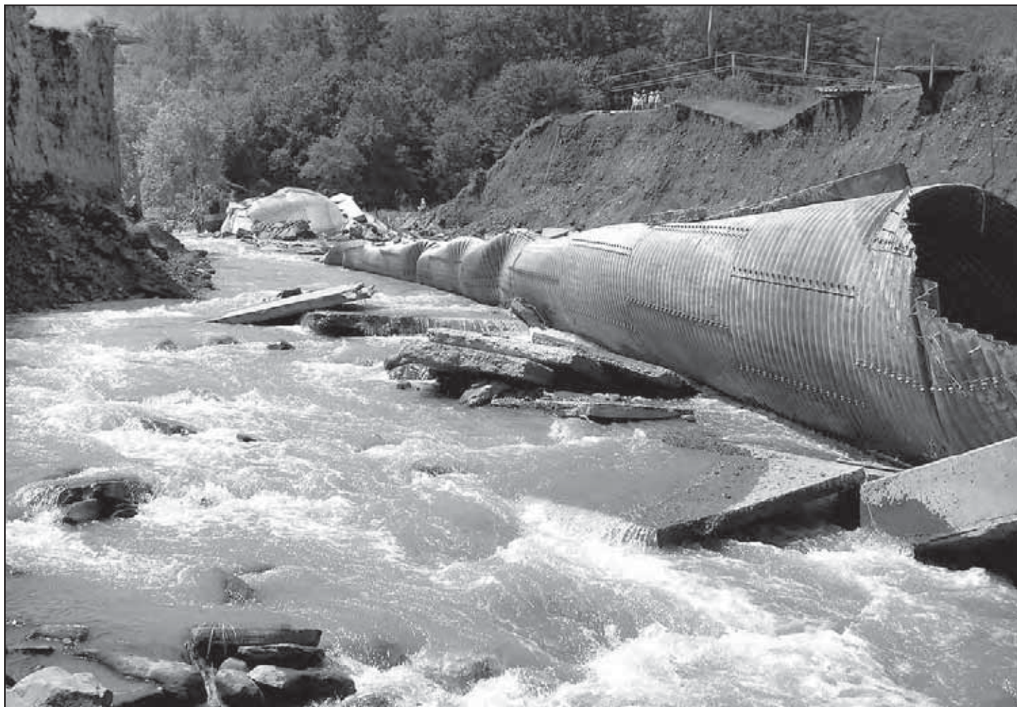
A view of the culverts that washed out under Interstate 88, near the Unadilla, NY exit as a result of heavy rains on June 29, 2006. Two truck drivers were killed driving into the collapsed highway.
