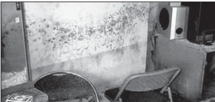
Example of mold spreading inside building affected by flooding.
