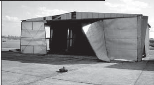
The Hammond municipal airport hangar damaged by Katrina winds.
