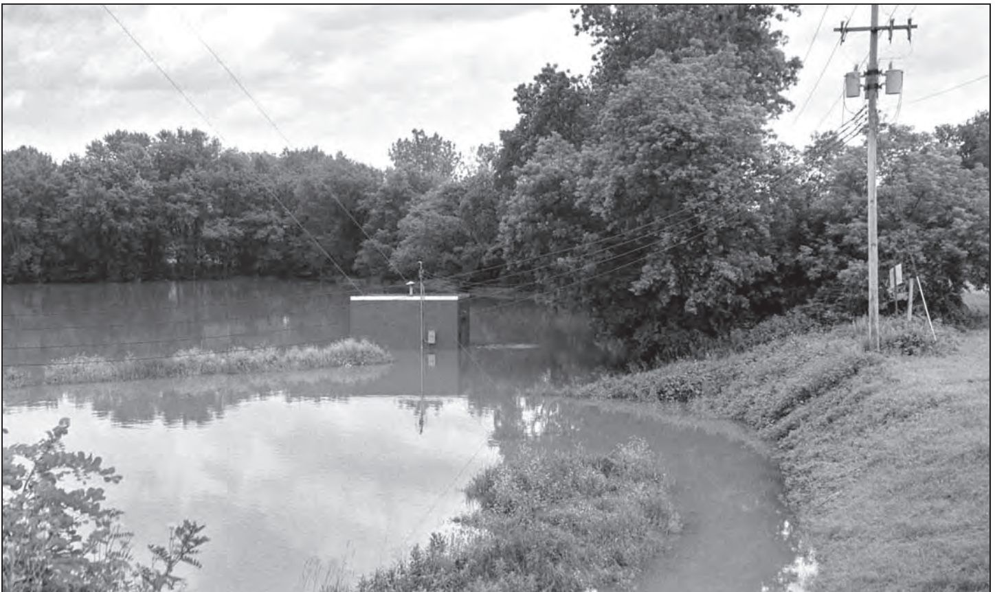
Nearby Town of Union's Frey Avenue pump station under water
