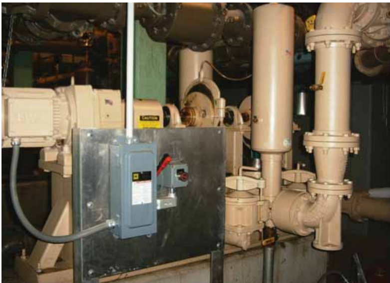
Plunger pump at Lake Placid WWTP
