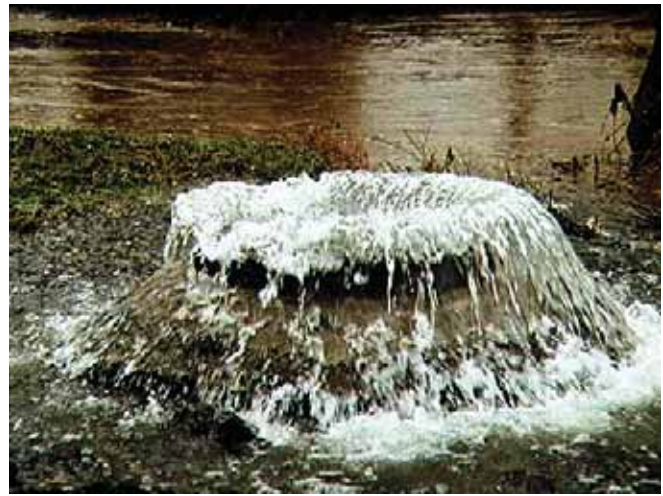
Many communities will have to pay for old sewer system failures.
