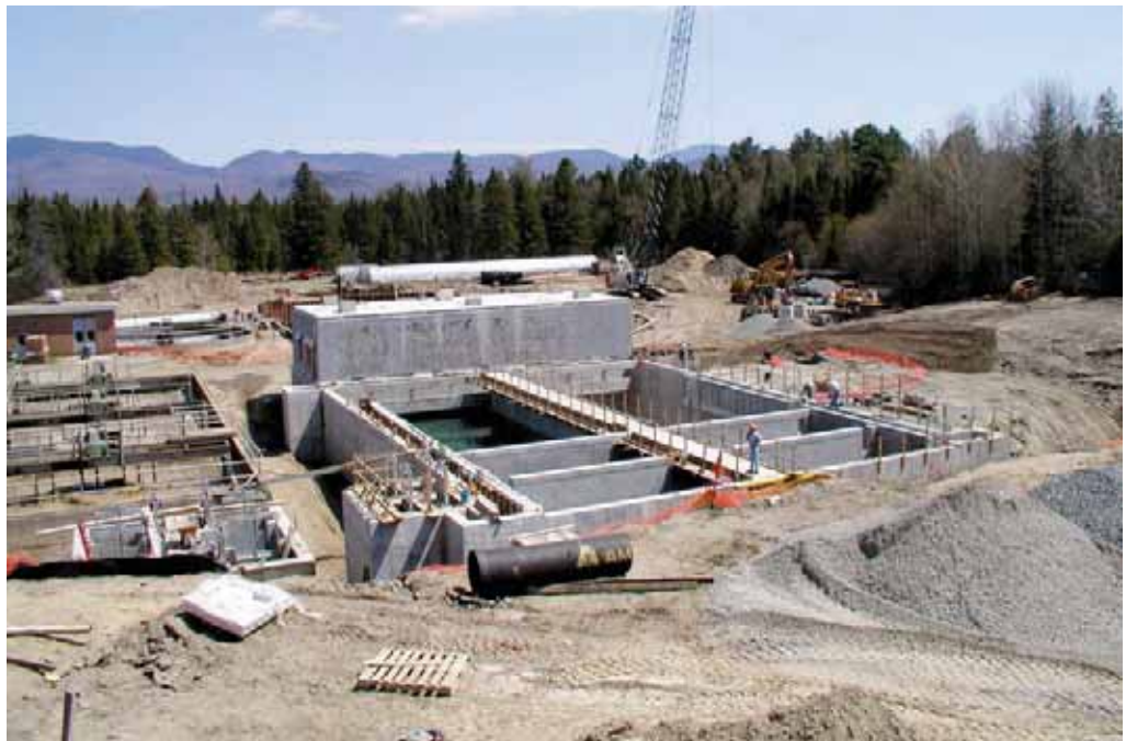
Sometimes a plant upgrade is needed to maintain SPDES compliance. (Lake Placid)
