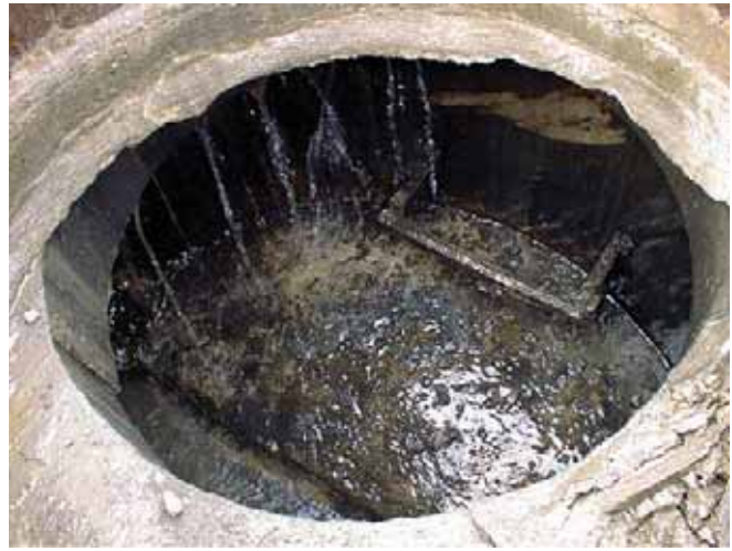
Groundwater infiltration makes efficient treatment difficult.
