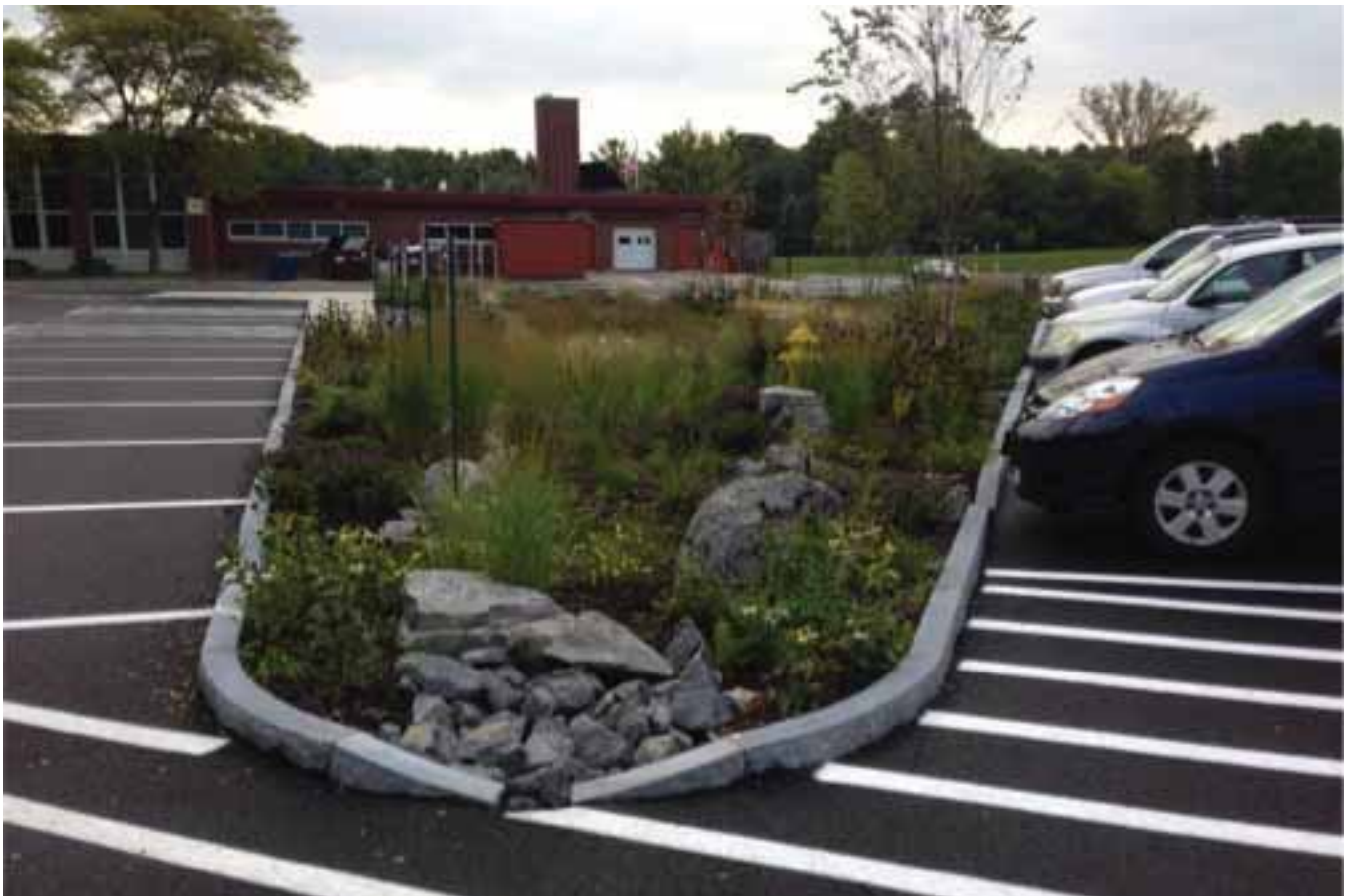
Rain garden at Mott Road Elementary School in Central New York
