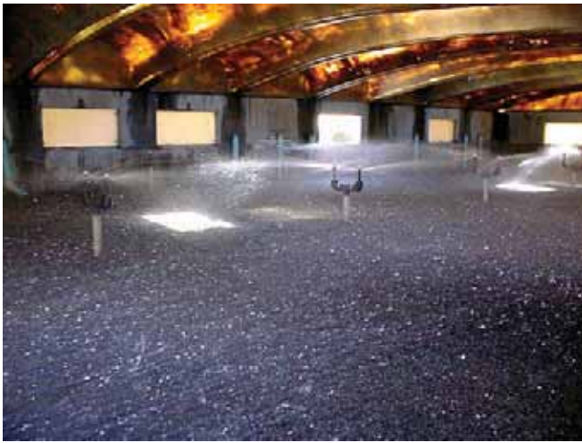
Intermittent sand filter (Secondary Treatment).
