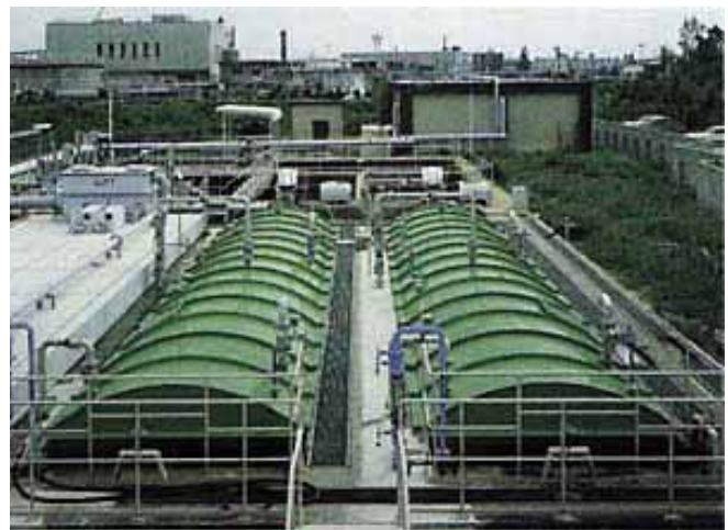
Sludge treatment and disposal is an important part of the process.
