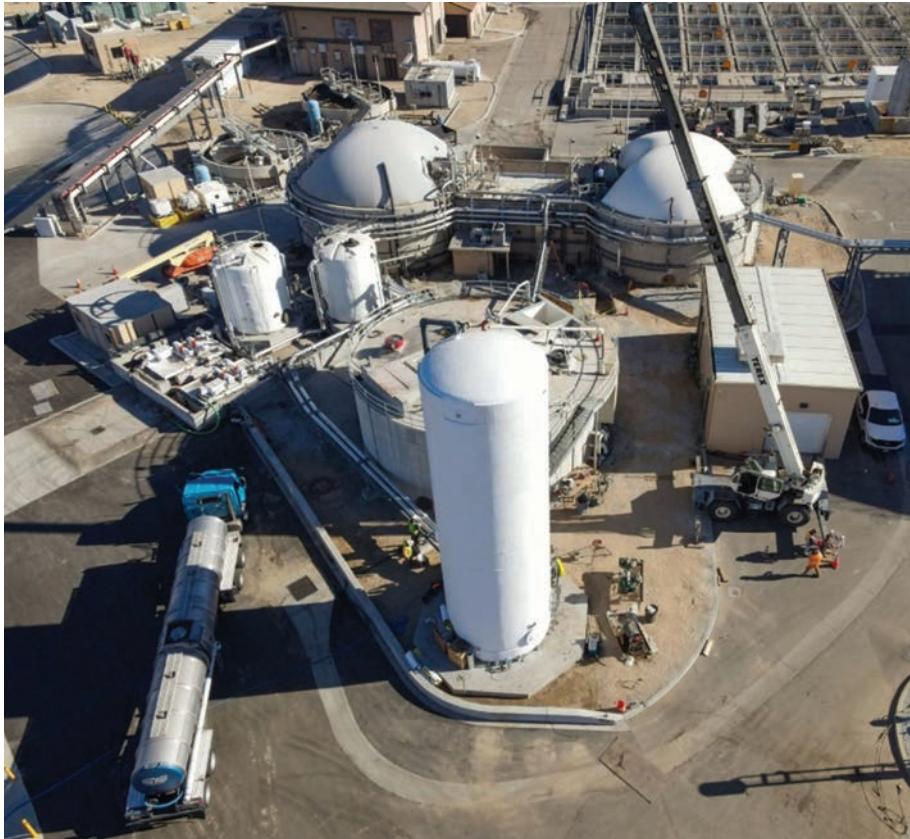
VVWRA establishes a landmark reference for biomethane production at any such wastewater resource recovery facility in the U.S. Anaergia
