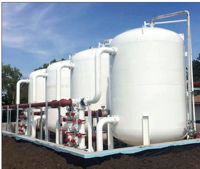
Figure 4. Granular activated carbon system for removing PFAS from drinking water in the State of Minnesota. Chow, et. al. 2022
