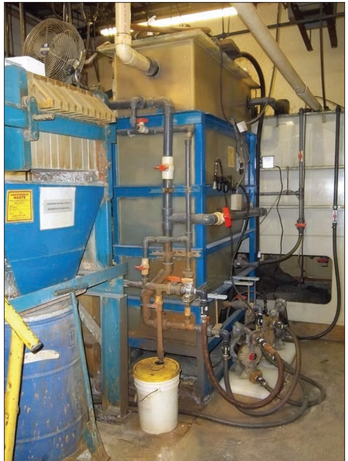
An example of a pretreatment plant at an industrial site.
