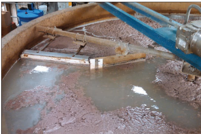
This dissolved air flotation system is one example of available pretreatment technologies.
