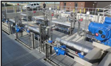
Bergen Point WWTP
