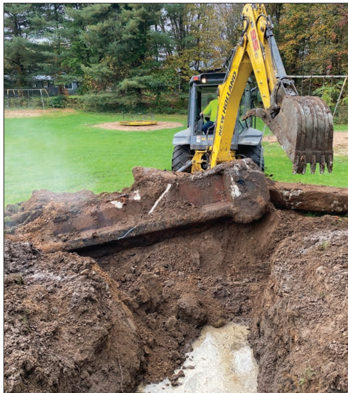
Digging up the stairs to the old school while looking for a water leak in the village park. David Hinds
