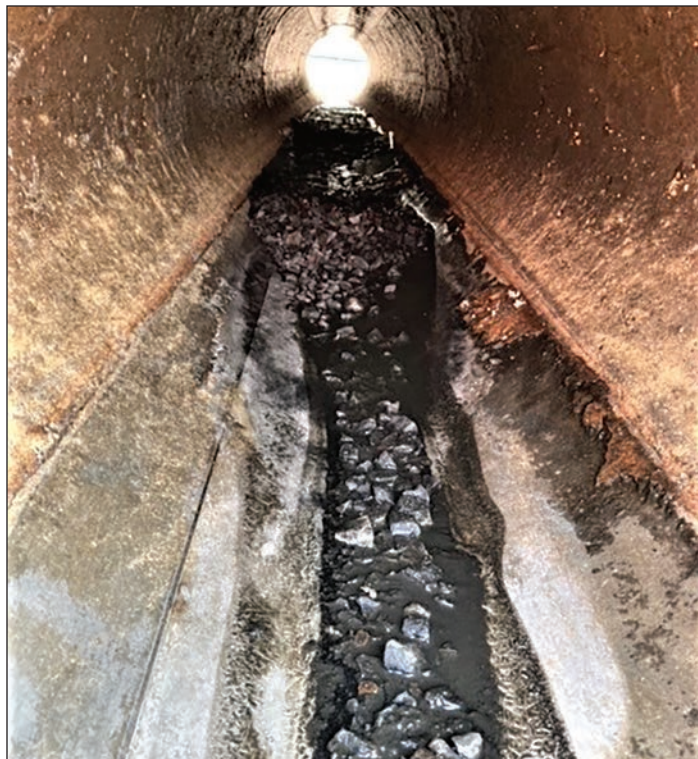
Photograph 3. View of the remaining construction stone in the 20-inch pipe (Aug. 9, 2021). Richard Kenealy
