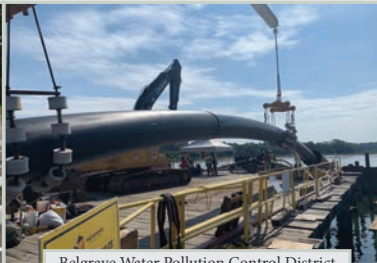
Belgrave Water Pollution Control District
