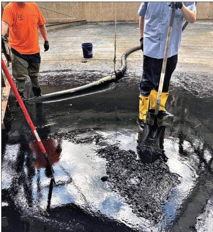
Photograph 2. Workers cleaning the construction stone from the bottom of FC#2 (July 30, 2021). Richard Kenealy
