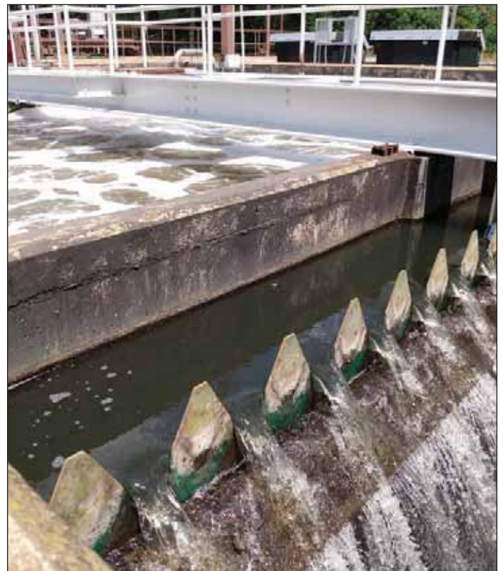
Diffused aeration replaced a 1970s mechanical mixer in the post aeration tank ahead of the effluent outfall during the effluent disinfection project in 2022. Michelle Hess
