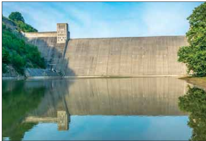
Mount Morris Dam and Recreation Area is a major flood control project and public park located on the Genesee River near the Village of Mount Morris in Livingston County, New York. The dam is situated deep in the Genesee River Gorge at the northern end of Letchworth State Park and provides flood protection to downstream areas including the city of Rochester. (Source: U.S. Army Corps of Engineers). Mike Haugh Photography
