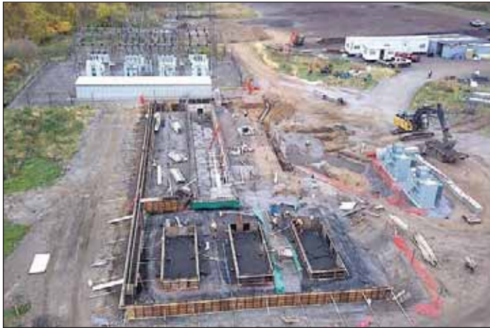
Construction progress drone photo of Electrical Building and RG&E substation, taken November 2022. Schuler-Haas Electric Corp.
