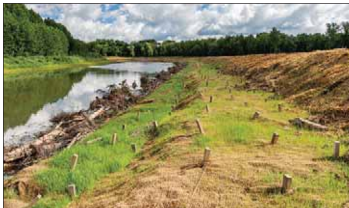
Chamberlain Property streambank stabilization project. Using a technique called a "toe-wood structure," large trees are placed at river bottom level and crisscrossed to form an inter-linked structure with the root wads pointed outward into the river current. Earth is backfilled over this assembly in two "bench" levels that are held in place by grass and tree plantings. Among other advantages, toe-wood projects improve habitat for fish and other aquatic life and provide a more natural appearance than rock-hardened structures. (Source: Genesee RiverWatch).
