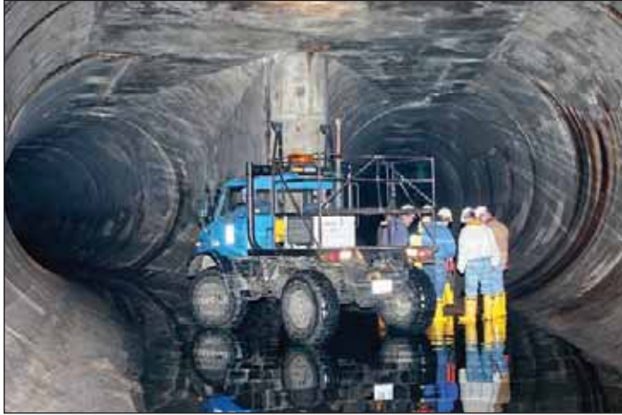
Monroe County DES staff touring the CSOAP Culver-Goodman Tunnel. Monroe County DES
