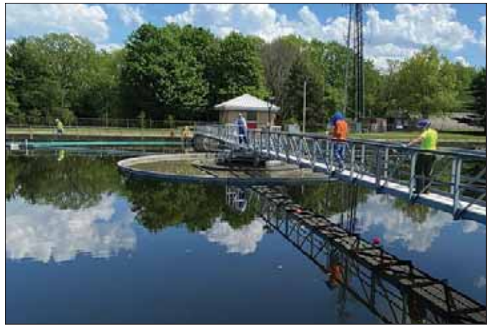
Field verification testing conducted by MCDES, Clarifier Performance Evaluations, Inc. and Arcadis staff. Hannah Rockwell/Arcadis
