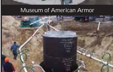
Courthouse Commons Pump Station
