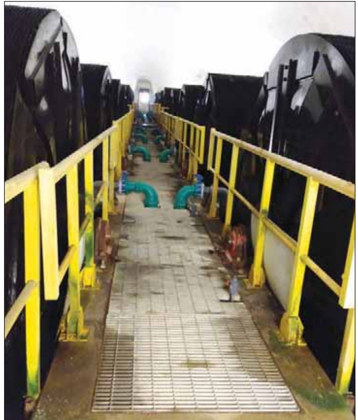
Sixteen RBCs quietly rotate in and out of the water providing enhanced biological treatment. Michelle Hess
