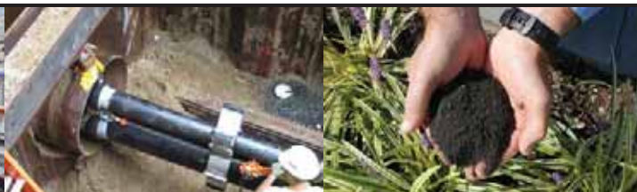
Ronkonkoma Hub Pump Station
