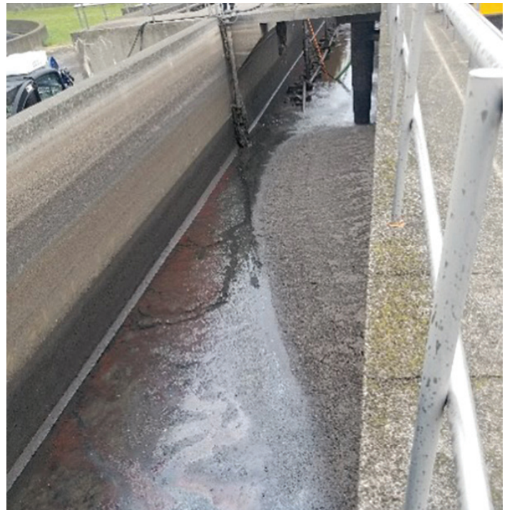
Figure 6. Bird Island WWTF aeration tank influent channel with accumulated grit and debris. AECOM
