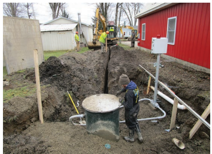
Simplex grinder installation.
