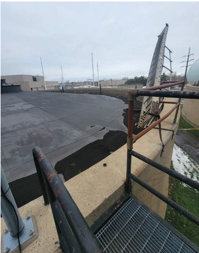
Digester tank with storm-damaged equipment, Dec. 29, 2022. Alex Emmerson, BSA
