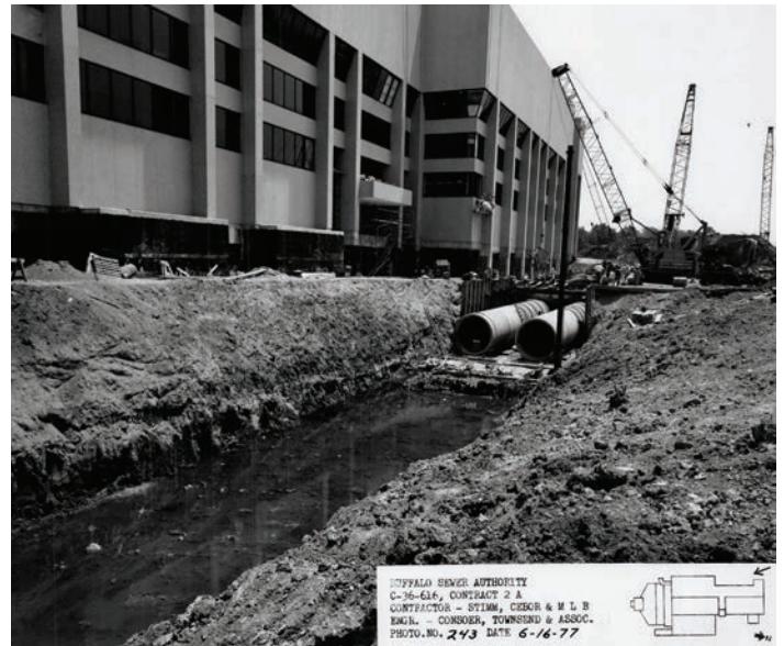
Figure 2. Construction photo of settled wastewater effluent pipes circa 1970s. Consoer, Townsend, & Associates via Buffalo Sewer Authority
