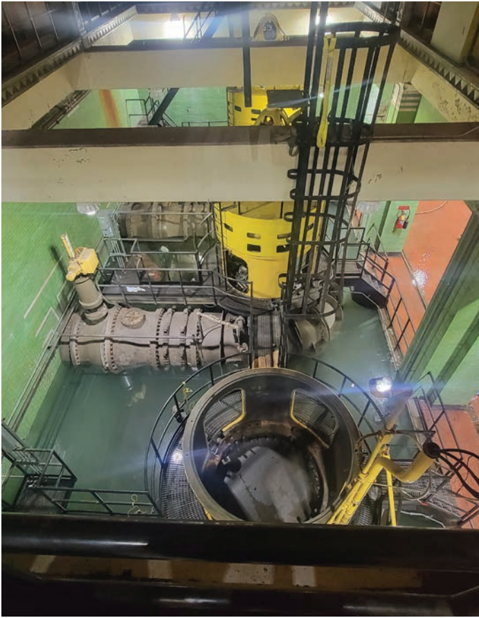
Flooding in the wastewater pumping station, Dec. 23, 2022. Alex Emmerson, BSA
