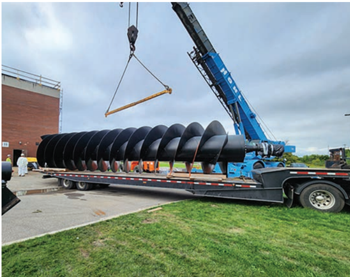
New 27.5 MGD influent Archimedes screw pump being moved into Southtowns AWTF. Erie County
