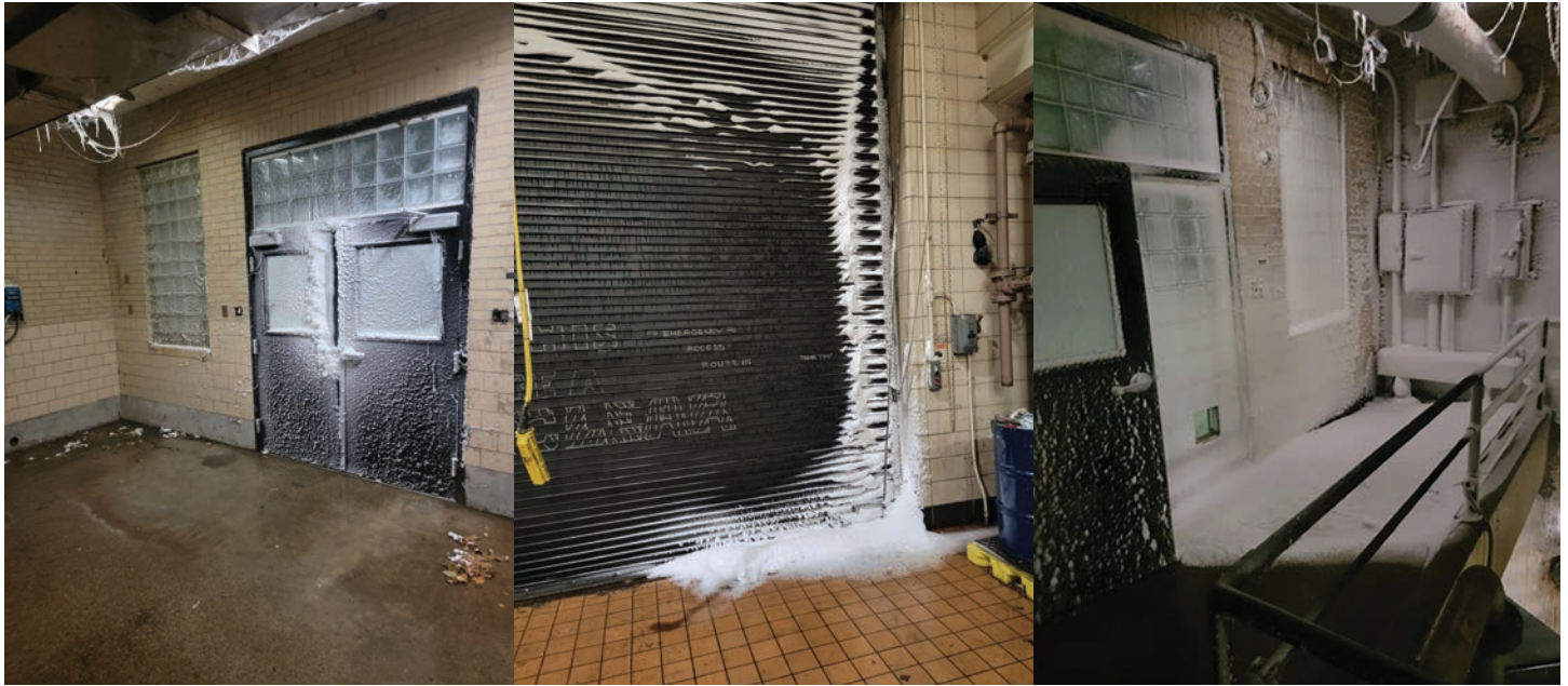
December 23, 2022. Left: Door seals were no match for the blowing snow. Middle: Louvered door with snow forced through by winds. Right: Snow inside building and over electrical panels came through a broken window. Alex Emmerson, BSA
