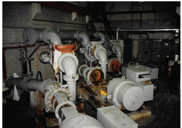
Figure 4. Pump room with 400-hp horizontal pumps in 1989. Rick Roll
