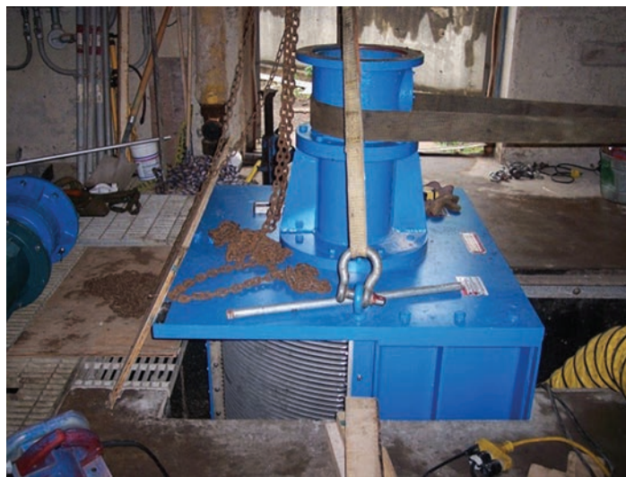
Figure 6. A crane lowers a new grinder into position, replacing manually cleaned bar racks. Rick Roll
