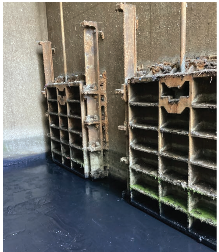
Figure 8. Bird Island WWTF chlorine contact tank sluice gates prior to removal. AECOM
