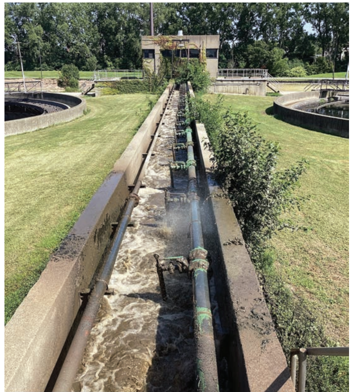
Figure 7. Bird Island WWTF final settling tank influent channel with damaged air header. AECOM
