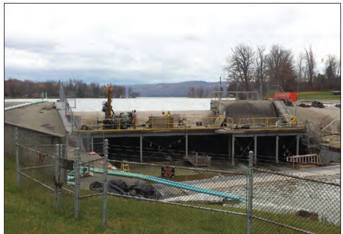
The Otisco Lake Dam during the construction phase. Visible in this image are the temporary siphons (blue pipes), the temporary support platform across the face of the dam, and the anchor drill rig. OCWA
