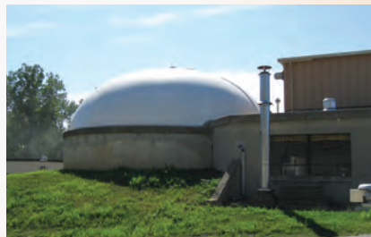
Digester Gas Holding Cover
