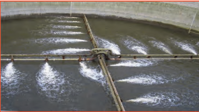
JET MIXING IN EQUALIZATION TANKS
