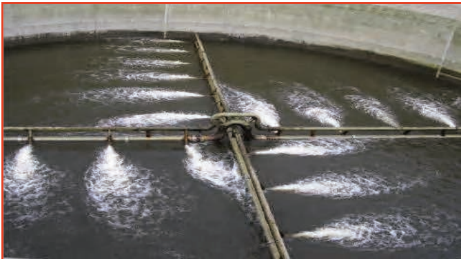
JET MIXING IN EQUALIZATION TANKS
