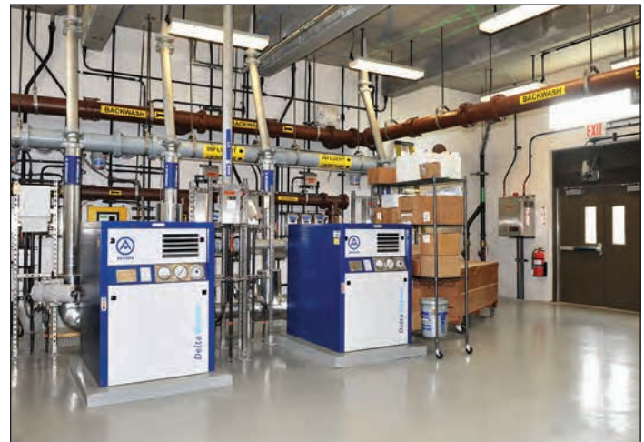
The denitrification system blends seamlessly with the existing infrastructure. Tony Lopez Photo
