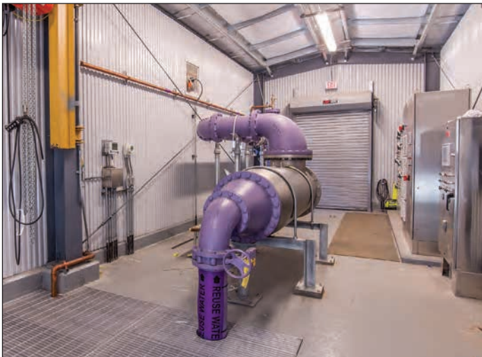
Reuse water supply piping to the golf course irrigation system, including a high strength ultraviolet disinfection vessel.
