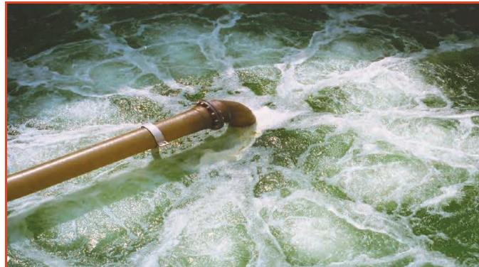
MIXING AND AERATION IN pH CONTROL TANK
