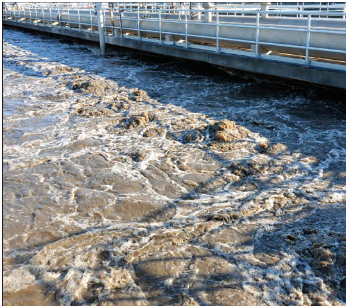
Aeration basins are one component of a nitrogen removal strategy at the Bay Park Sewage Treatment Plant. istockphoto.com
