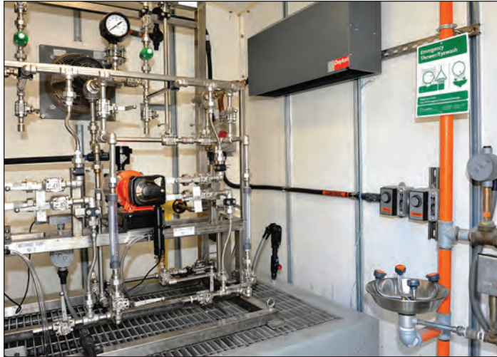
Chemical metering pumps precisely regulate the amount of methanol infused into the denitrification system. Tony Lopez Photo
