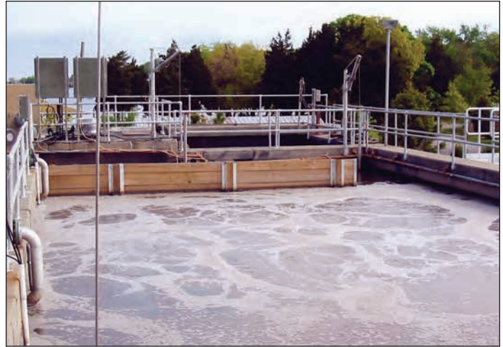
The aeration tank and anoxic zone baffles are an integral part of the MLE process. Gannett Fleming
