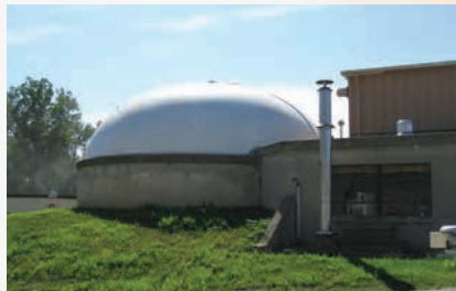
Digester Gas Holding Cover
