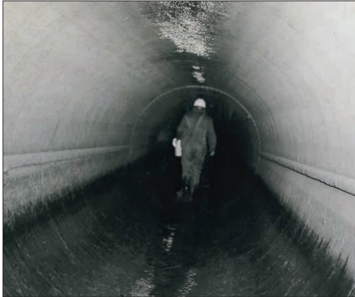
Figure 3. An inspector walks through the pipe in Seaford, Manhole No. 19, during inspection of the 72-inch steel force main of the Sunrise Highway Aqueduct System in 1977. Nassau County Department of Public Works
