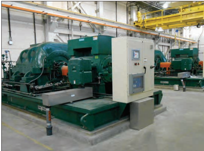
Four new blowers were installed in the air process system of the Tallman Island Wastewater Treatment Plant in College Point.
