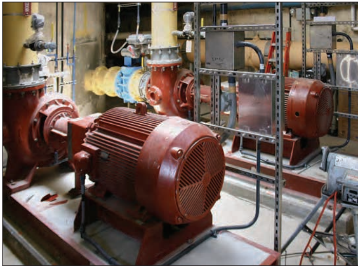
A mixed flow pump station was rehabilitated at the Tallman Island Wastewater Treatment Plant in College Point.
