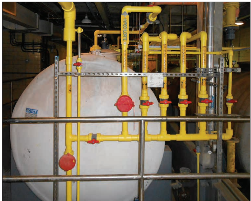
One of the upgrades to the Tallman Island Wastewater Treatment Plant in College Point is a new sodium hypochlorite tank and delivery system.
