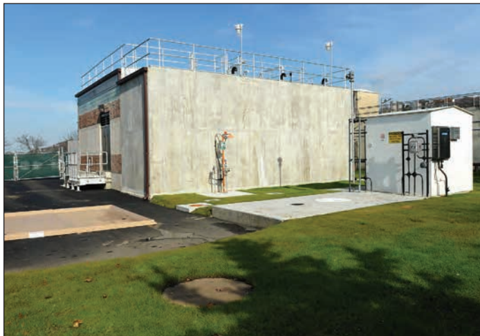
The denitrification facility is the heart of the upgrade project. Tony Lopez Photo
