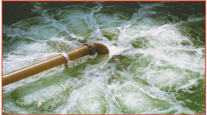
MIXING AND AERATION IN pH CONTROL TANK
