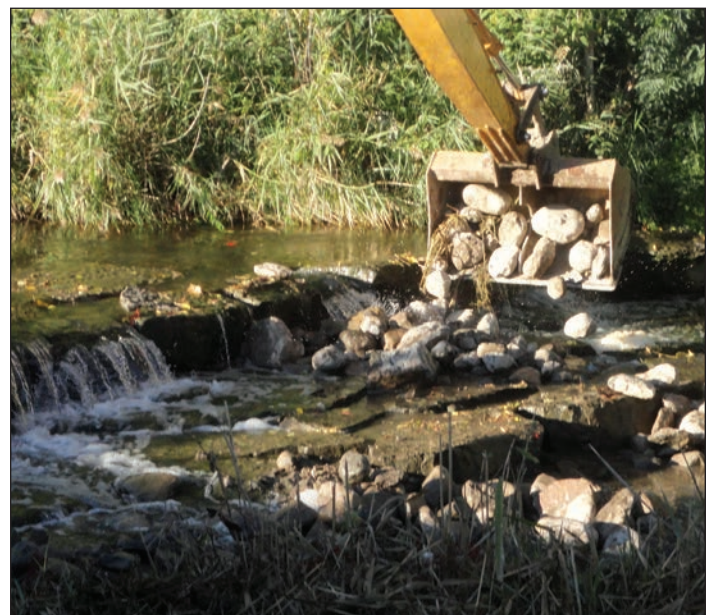
Photograph 2. Heavy equipment is used to place stone fill on and downstream of the dam structure in the South Branch of Ley Creek near Tarbell Road. Les Monostory
