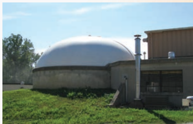
Digester Gas Holding Cover
