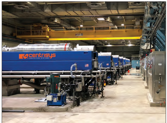
New dewatering centrifuges at Wards Island Water Resource Recovery Facility. NYCDEP
