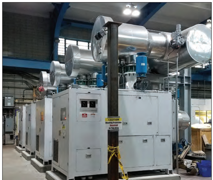
New turbo process air blowers at 26th Ward Water Resource Recovery Facility. NYCDEP
