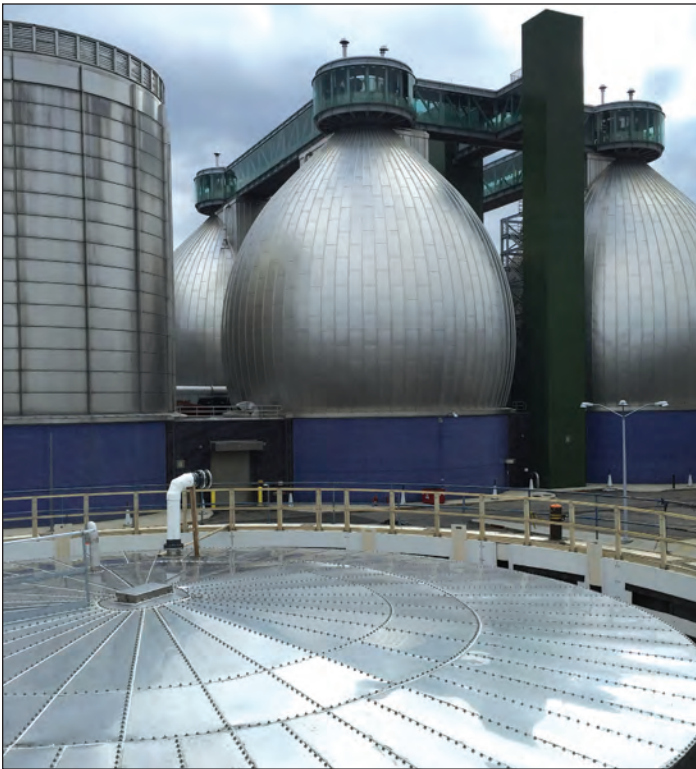
Food waste storage tank and digester eggs at the Newtown Creek Water Resource Recovery Facility. NYCDEP
