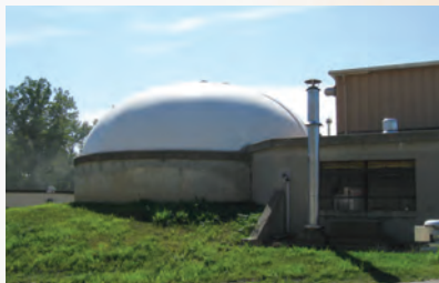
Digester Gas Holding Cover
