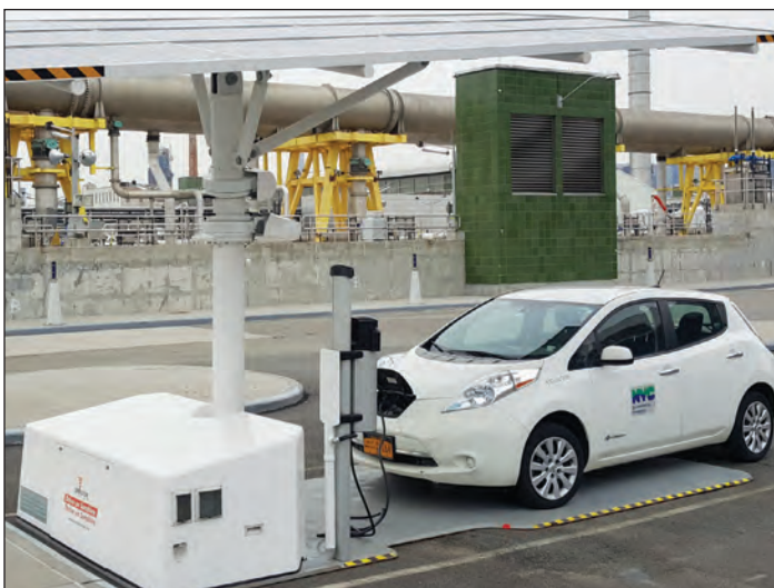
Solar carport portable electric vehicle charging station at Newtown Creek Water Resource Recovery Facility. NYCDEP
