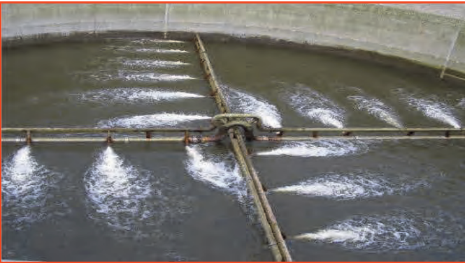
JET MIXING IN EQUALIZATION TANKS
