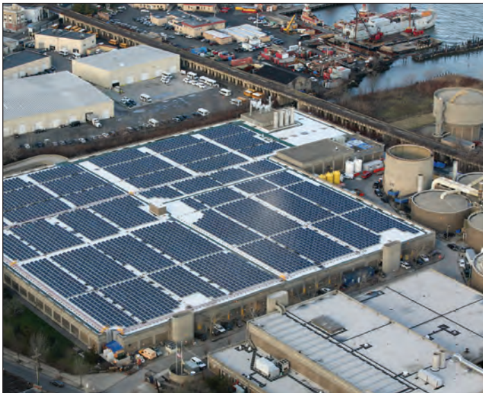
Solar PV system at Port Richmond Water Resource Recovery Facility. NYCDEP
