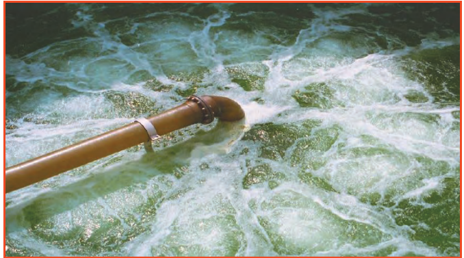
MIXING AND AERATION IN pH CONTROL TANK
