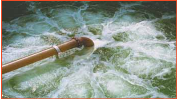
MIXING AND AERATION IN pH CONTROL TANK
