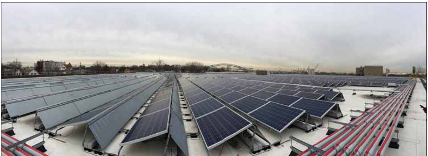
Solar panel installation at Port Richmond Wastewater Treatment Plant in Staten Island.
