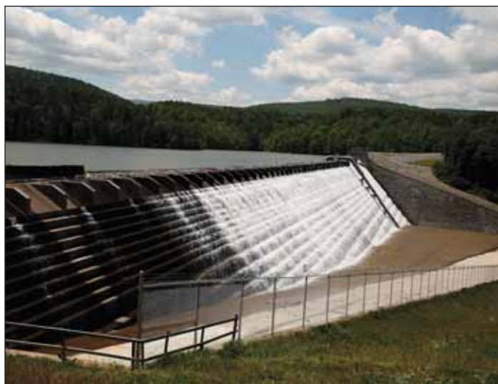
Gilboa Dam after rehabilitation, July 2015. The steps help to dissipate the energy of the water. New York City DEP
