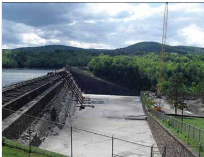
Gilboa Dam at the Schoharie Reservoir before rehabilitation, May 2010. New York City DEP
