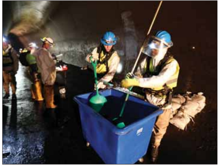
The interior lining of the 74-mile-long Catskill Aqueduct is being scrubbed to decrease friction, which will increase the tunnel’s capacity by approximately 30 to 40 million gallons of water each day. New York City DEP
