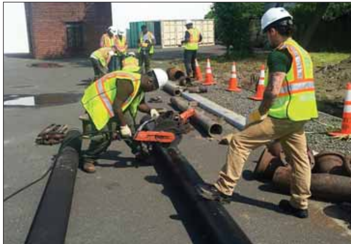
An Apprentice Construction Laborer learns safe operation techniques for operating a circular saw. New York City DEP
