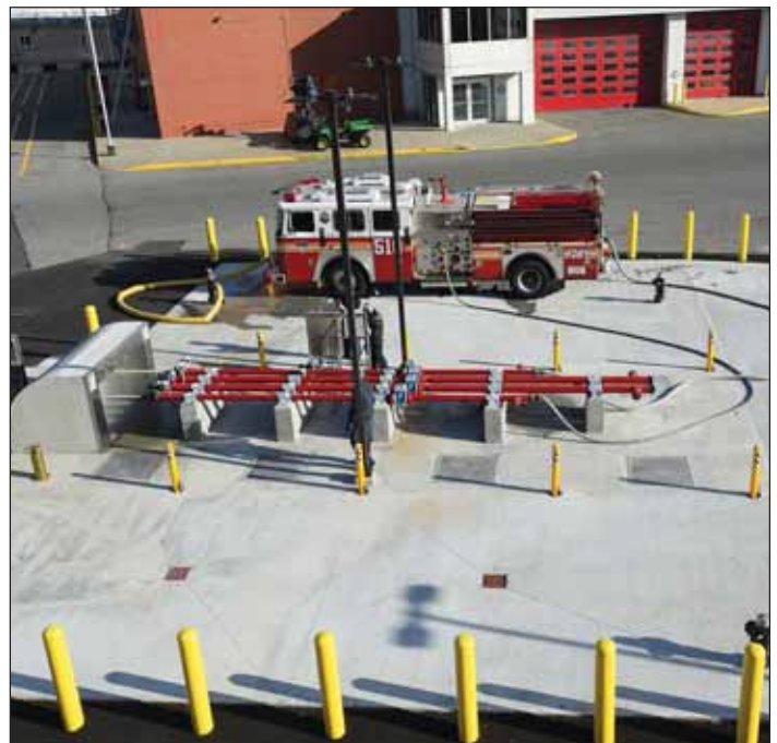
A 40,000-gallon storage tank and water recovery facility at the Fire Department training facility on Randall's Island collects used water in an underground tank and reuses it to calibrate equipment used on fire trucks.
