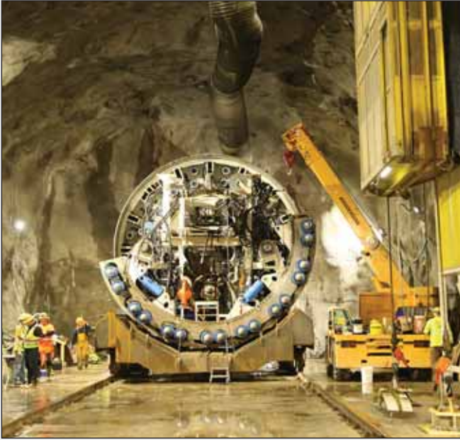
Back of the cutter head support, Delaware Aqueduct repair. New York City DEP
