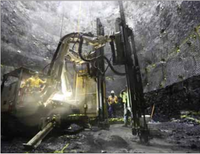
Shaft 5b, in Newburgh, New York, was constructed using drill and blast techniques as part of the Delaware Aqueduct repair project. This shaft will serve as the TBM launch site. A similar shaft at Wappinger, New York, will serve as the TBM retrieval site. Kristen Artz, New York City DEP
