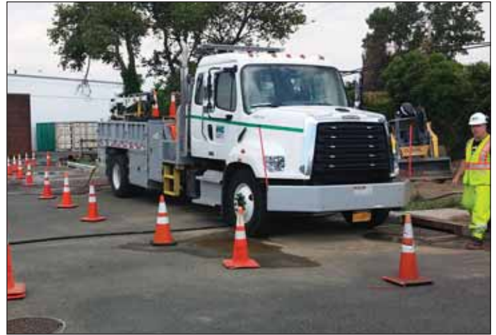
At the Bureau of Water and Sewer Operations Field Training Center, the Apprentice Construction Laborers learn how to set up a safe work zone.
