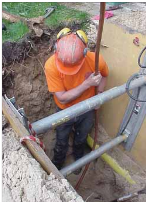
Staff of the Madison Water Utility replacing lead pipe as part of their Lead Service Replacement Program.
