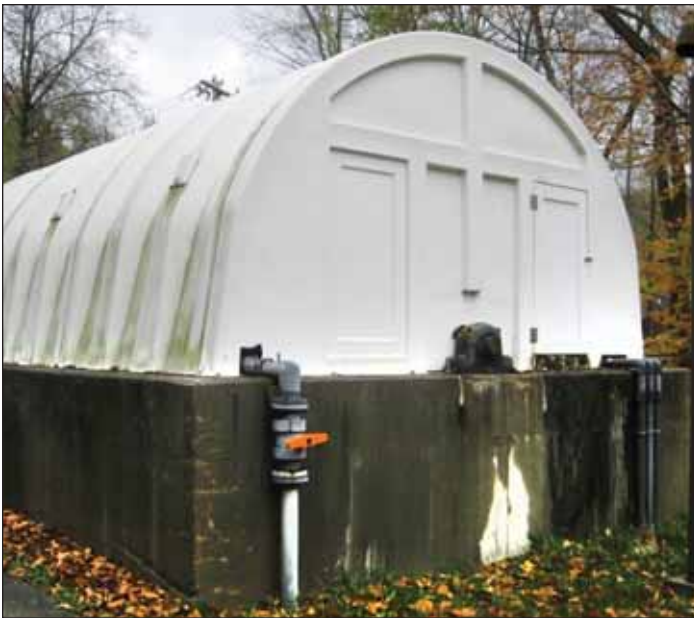
Figure 3. Photographs are another means to monitor municipal assets, such as this condition assessment of the RBC tank cover at Carmel Sewer District No. 4. NYSDEC
