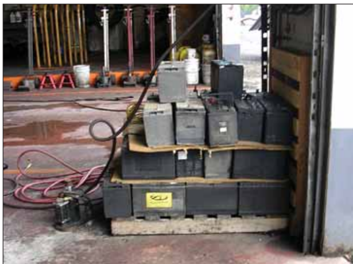
Open battery storage is more an employee hazard than a release issue, especially in high traffic areas. OBG
