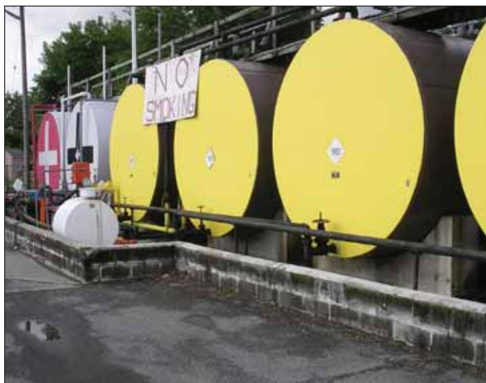
Practices related to above ground tanks should be scrutinized carefully for release potential, now or in the past. OBG
