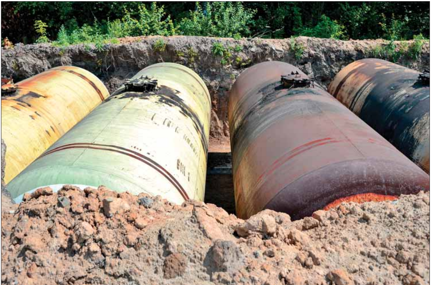
Forgotten underground storage tanks are one of many potential concerns that a Phase I ESA may find on a subject property.
