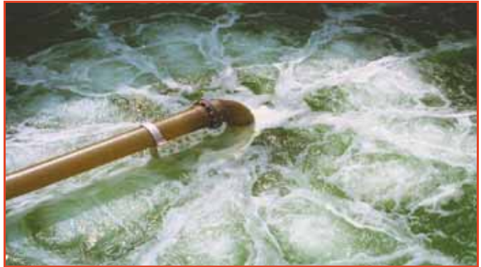
MIXING AND AERATION IN pH CONTROL TANK
