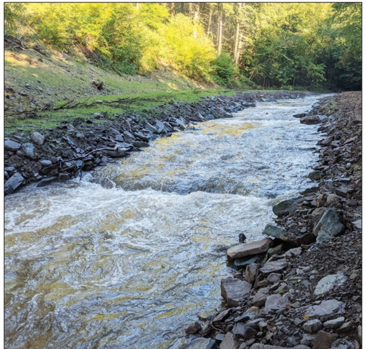
The completed project on Steele Brook included loose stones placed along the stream edges to slow the stream and reduce potential damages downstream. November 2021.
