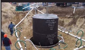
Courthouse Commons Pump Station
