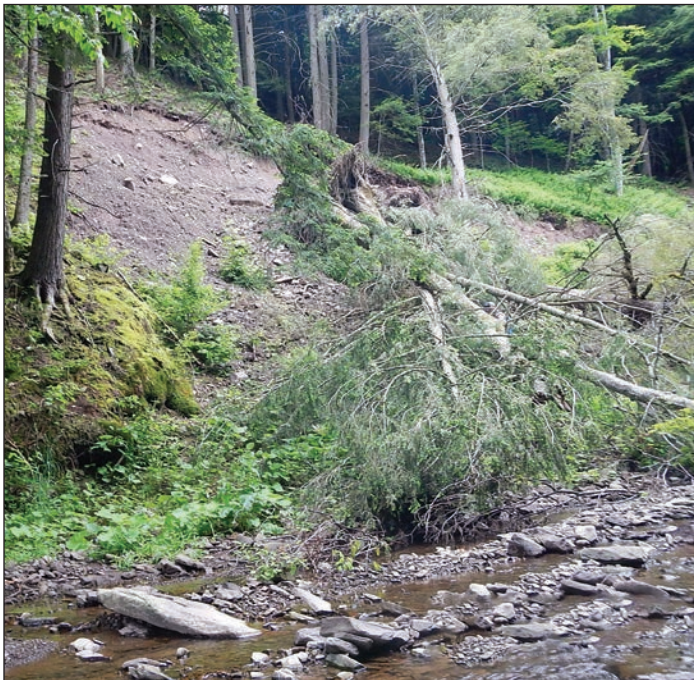
As part of the project, the fallen trees and debris needed to be cleared from Steele Brook and its 21-foot-high sloped banks. June 2017.
