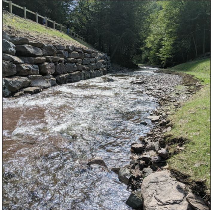
The completed project on Steele Brook, which includes a stacked rock wall to retain the slope and reduce sediment loading to the stream during storm events. November 2021.
