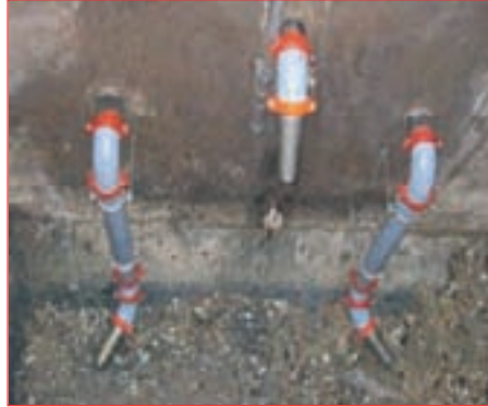
NOZZLES BEFORE OPERATION
