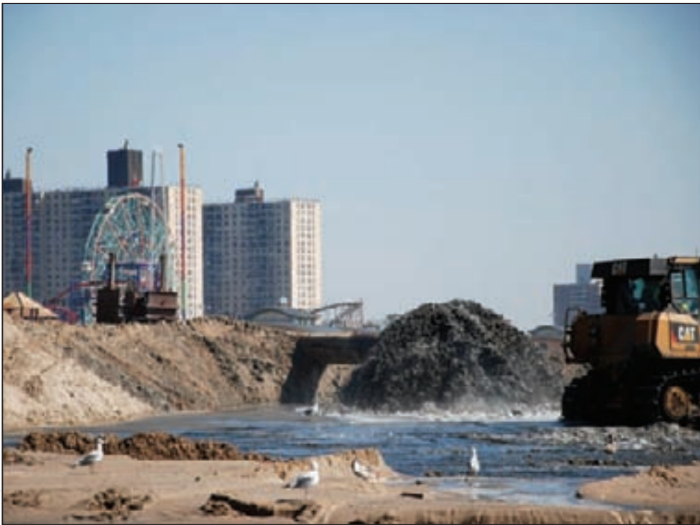
Close up of sand being pumped onto the beach of Coney Island, NY
