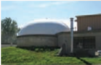
Digester Gas Holding Cover
