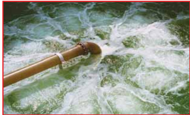
MIXING AND AERATION IN pH CONTROL TANK
