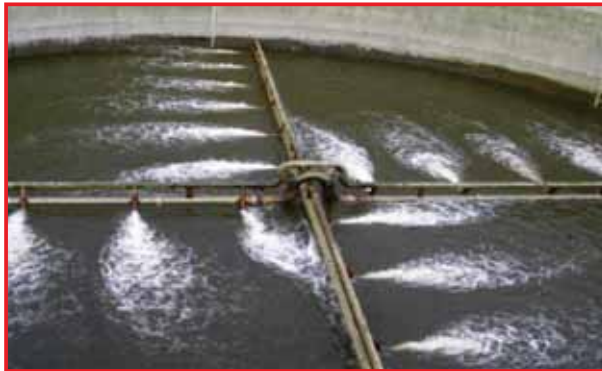
JET MIXING IN EQUALIZATION TANKS
