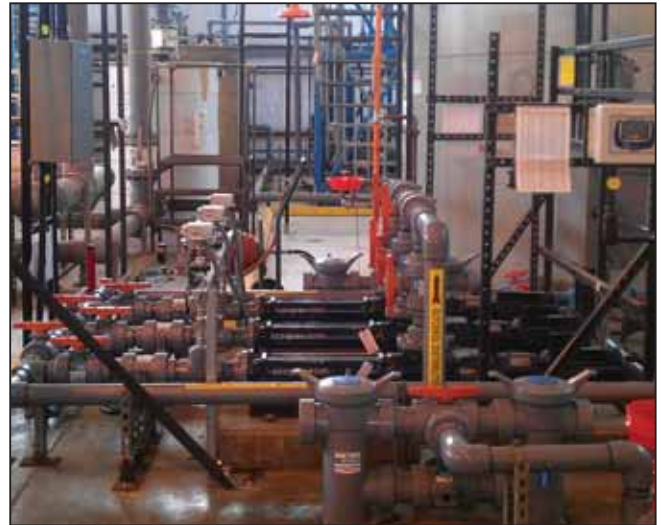
The glycerol addition system that services the SCT process consists of three progressive cavity pumps, a network of piping, various meters and sensors, and two storage tanks (one storage tank is visible in right background).
