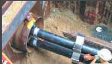
Ronkonkoma Hub Pump Station
