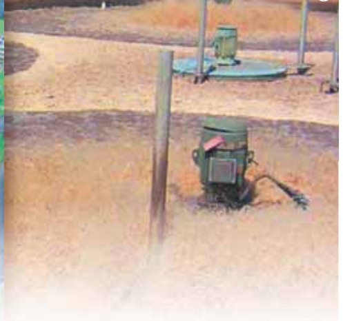
Aeration and Mixing
