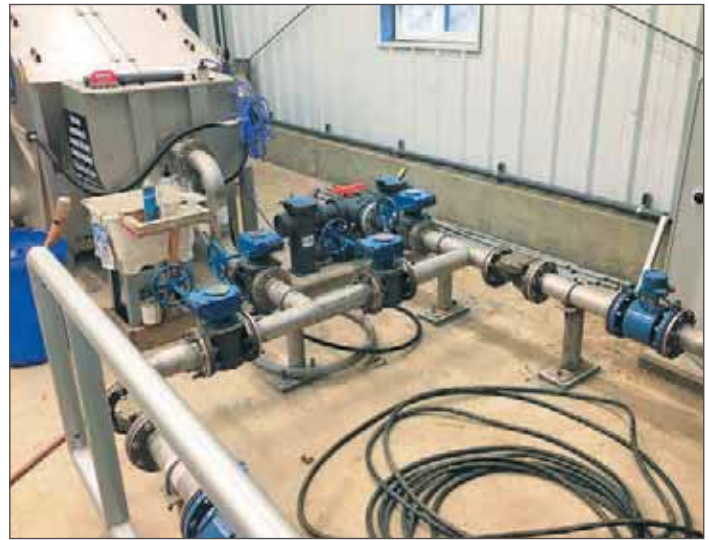
HSOW screen and influent piping with flow meters. Amy Hait/B&L
