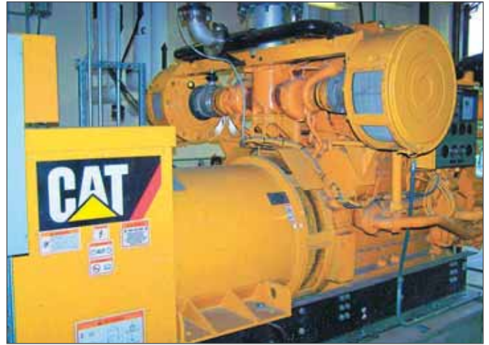
GJJWTF's combined heat and power (CHP) generator producing electricity from co-digestion. George Bevington, B&L
