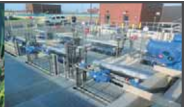
Bergen Point WWTP
