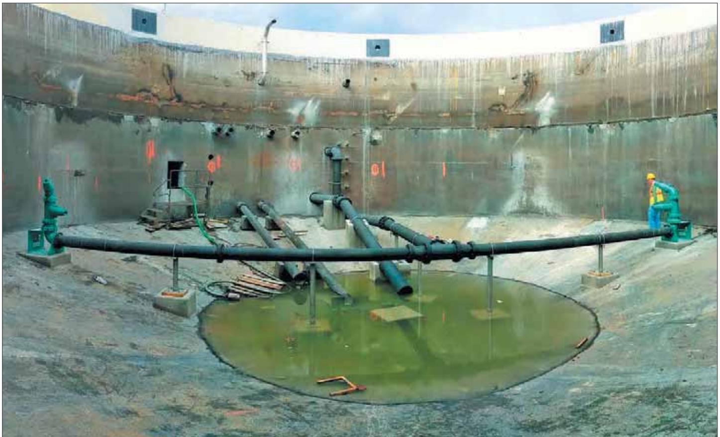
Inside Digester 2 with pump and nozzle mixing system.
