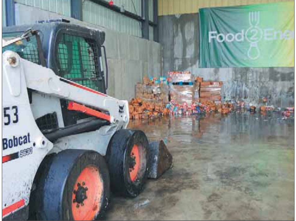
Preparing to load packaged food into the depackaging unit at the OHSWA Food2Energy Facility. Christian Glander, NYSDEC
