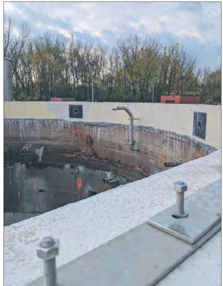
Cold joint along Digester 2.
