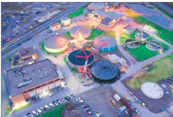
Metropolitan Syracuse Wastewater Treatment Plant Sludge Dewatering Complex Construction. Onondaga County Department of Water Environment Protection
