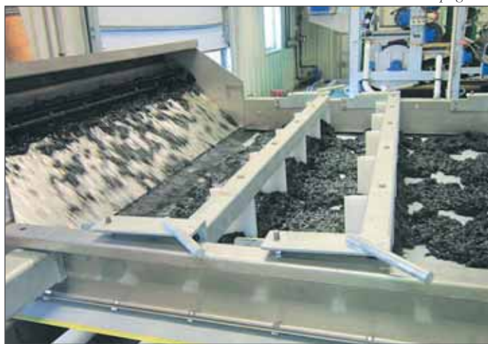
The City of Niskayuna WWTP gravity belt thickener for recuperative thickening.
