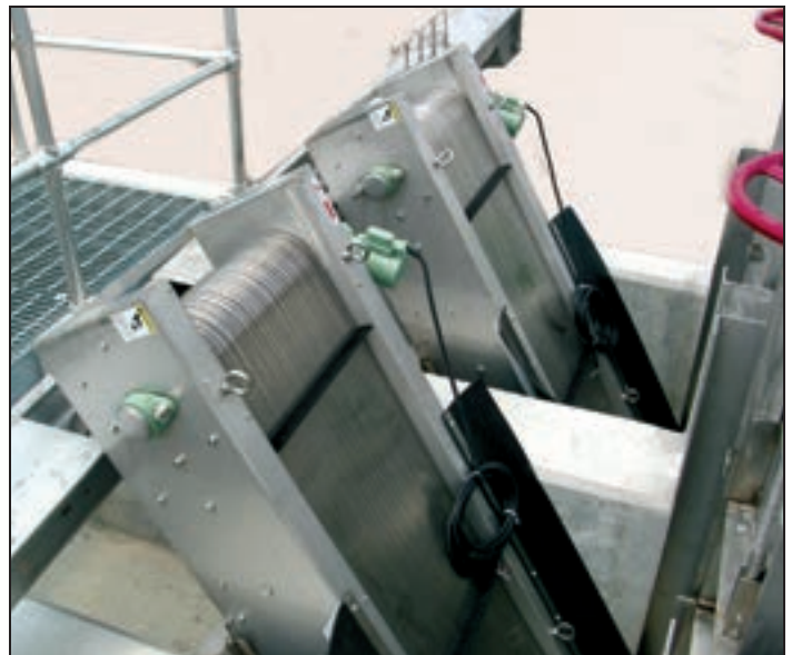
Figure 6. Dual fine screen system shown installed in concrete channel.
