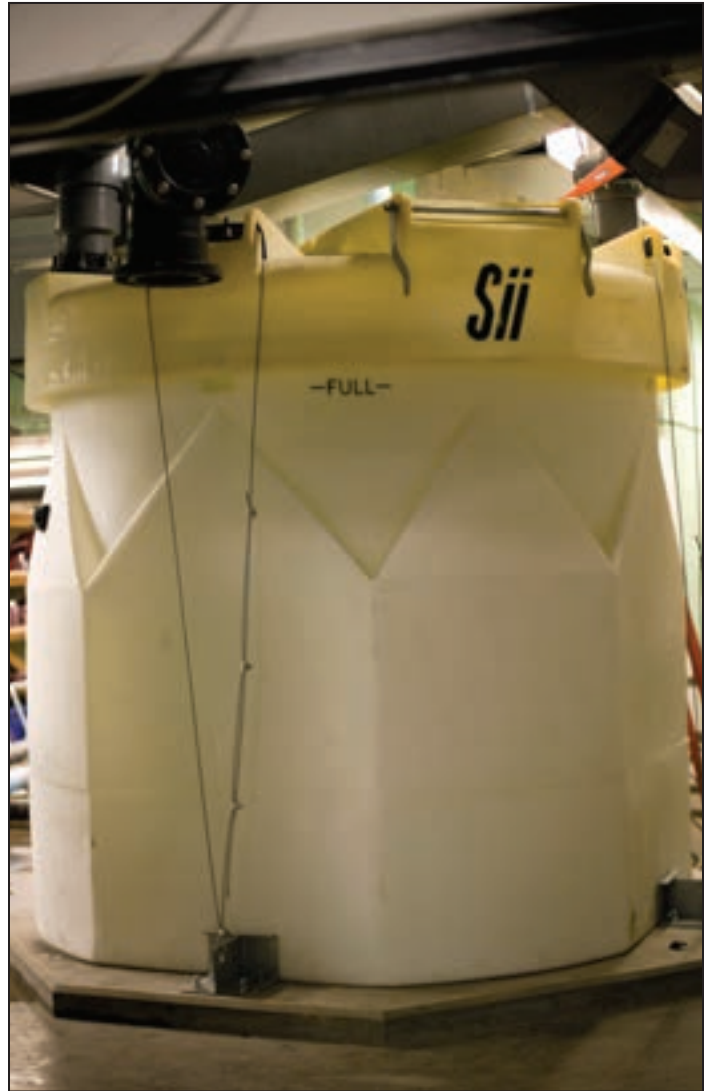
War Memorial Arena stormwater re-use cistern system
