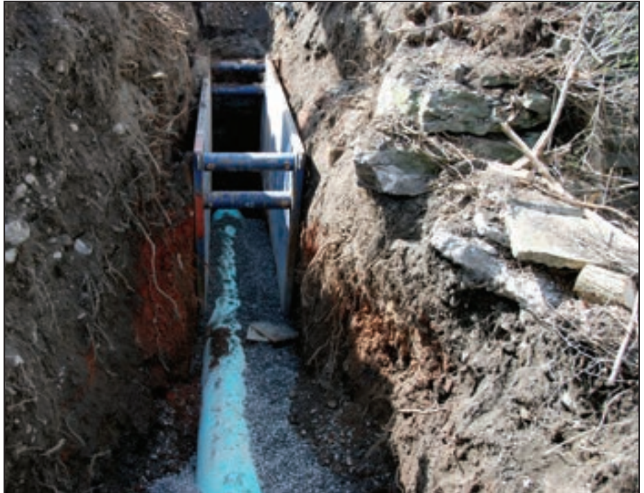
This photo shows an expensive repair taking place on a leaky sewer line in a municipal system.
