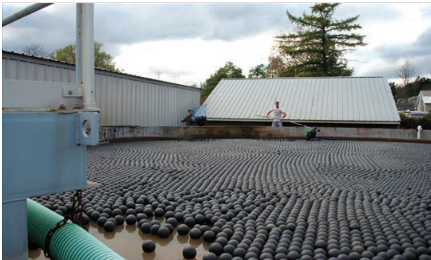
Plastic balls placed on top of an activated sludge bioreactor tank at a pharmaceuticals wastewater treatment plant form a floating insulation blanket helping to retain temperatures.
