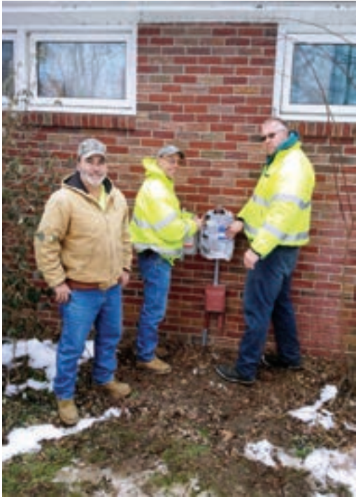
Town of Pendleton Water/Sewer Superintendent Jim Argo (far left), along with Pendleton Field Technicians Jeff Jarvis (center) and Rick Geltz (right), with one of the Town's 400 E/One Upgrade grinder pump control panels.
