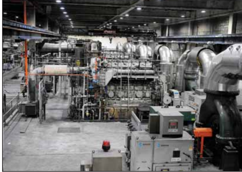
These North River WWTP direct-drive engines will soon be replaced by engine generators to achieve higher fuel efficiency and a reduced carbon footprint. Image courtesy of NYCDEP
