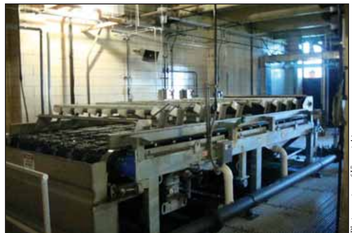
Figure 3. Two gravity belt thickeners (GBTs) are installed in the Main Sludge Disposal Building.
