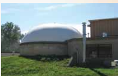
Digester Gas Holding Cover
