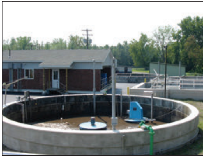
Village of Weedsport Wastewater Treatment Plant’s sequencing batch reactors
