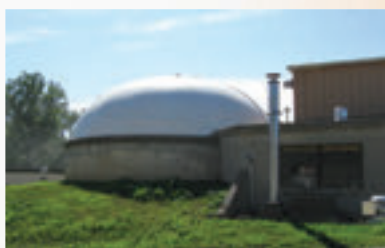
Digester Gas Holding Cover
