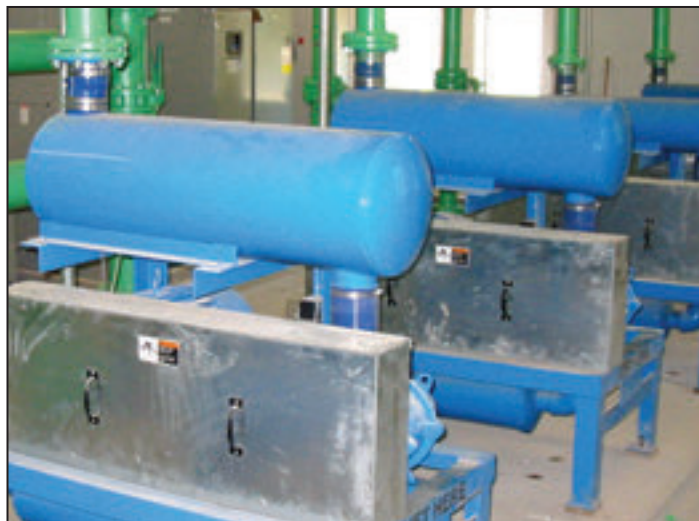
An example of the treatment plant's assets include these sequencing batch reactor blowers.
