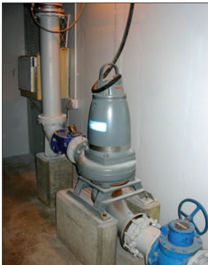
Assets at the plant, like this pump, are maintained and serviced at regular intervals, and all work recorded on CMMS software.
