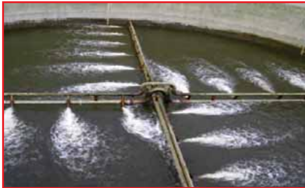
JET MIXING IN EQUALIZATION TANKS
