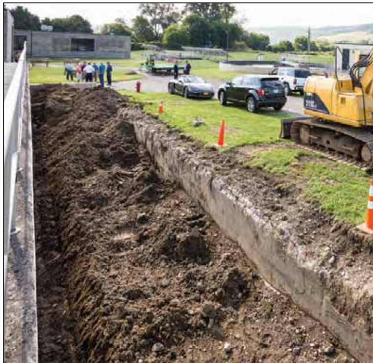
Workers remove part of the structure of the Hornell Water Pollution Control Plant to make room for a new blower building to be constructed.
