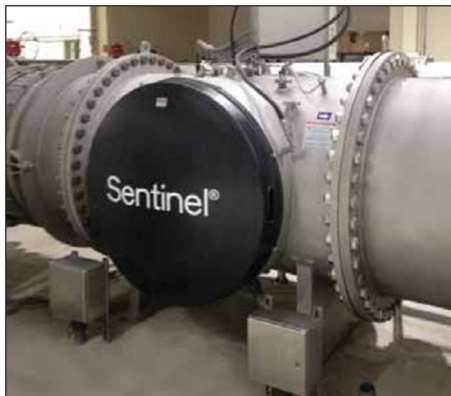
Figure 2. UV AOP system used to treat pollutant NDMA for potable reuse
