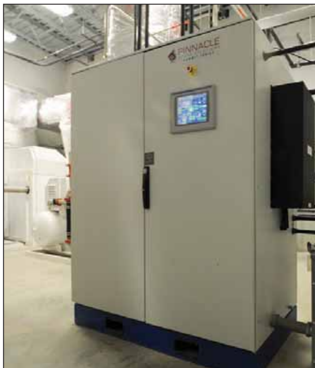
Installed Pinnacle system at Emmons, ND, water treatment plant
