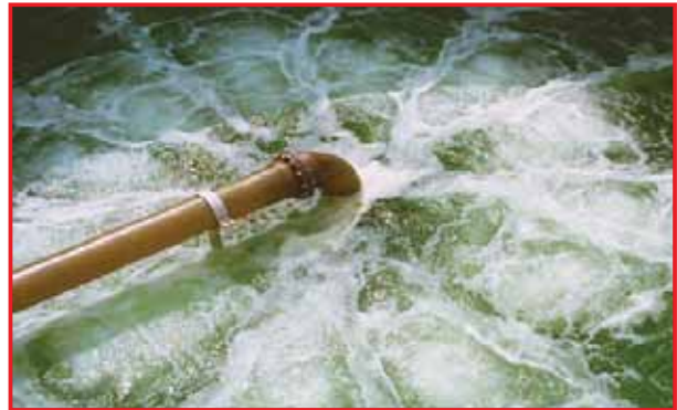
MIXING AND AERATION IN pH CONTROL TANK
