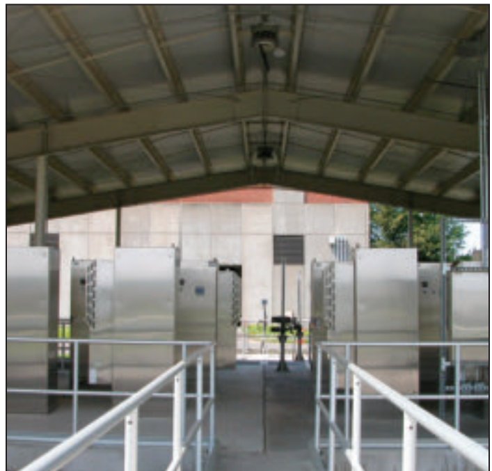
The ACSD South Plant’s four-channel Wedeco Duron ultraviolet system
