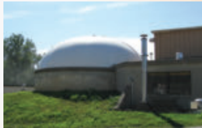
Digester Gas Holding Cover
