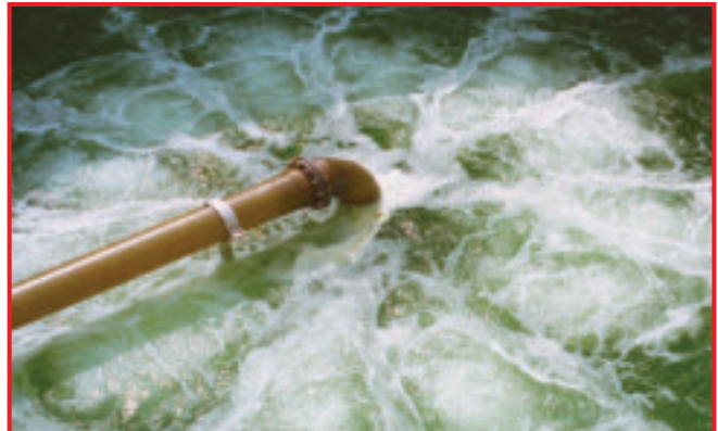
MIXING AND AERATION IN pH CONTROL TANK
