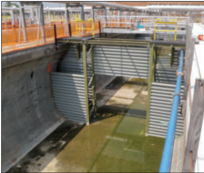
Figures 7A and 7B. Aeration tank upgrades to accommodate BNR (biological nitrogen removal) at the Jamaica Bay plant: froth hoods (top) and overflow/underflow baffles (bottom)
