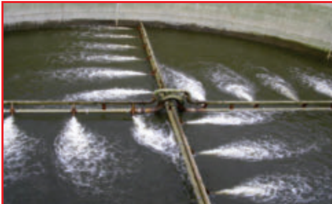
JET MIXING IN EQUALIZATION TANKS
