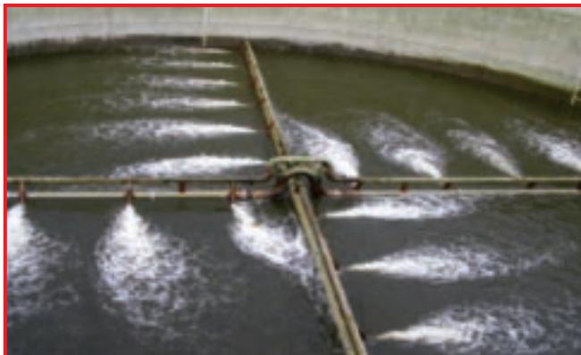
JET MIXING IN EQUALIZATION TANKS
