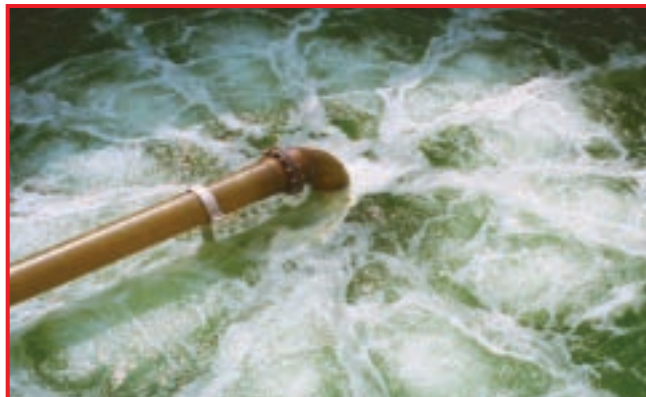
MIXING AND AERATION IN pH CONTROL TANK
