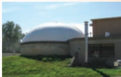
Digester Gas Holding Cover
