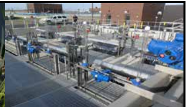
Bergen Point WWTP
