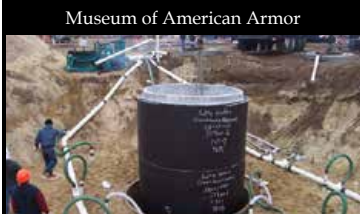
Courthouse Commons Pump Station
