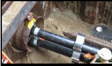
Ronkonkoma Hub Pump Station
