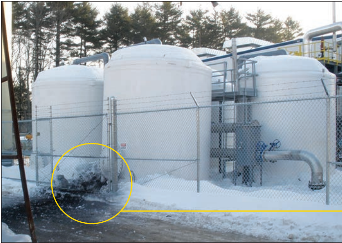
Photograph 1. A carbon absorber failed catastrophically within five days of startup, when the anchor system failed, and bottom blew out.
