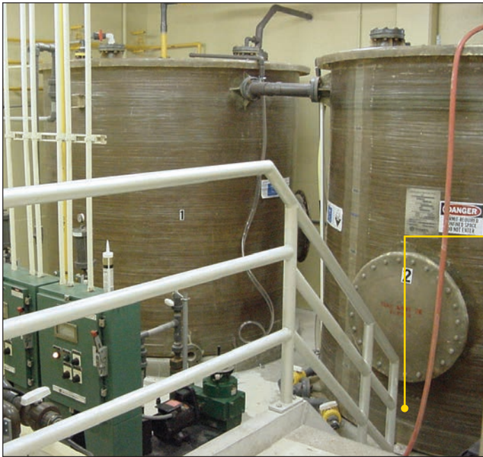
Photograph 5. Pair of sodium hypochlorite tanks that were replaced after seven years of service due to excessive FRP deterioration and through-wall leakage.
