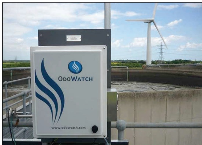
Figure 4: Electronic odor monitoring system.
