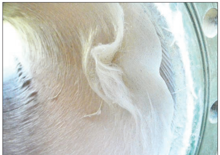
Photograph 1. In this case, a less expensive polyester resin was used by mistake in a part of ductwork fabricated for odor control in a wastewater treatment plant. The resin was attacked by sulfuric acid and the FRP laminate failed. Randy Nixon
