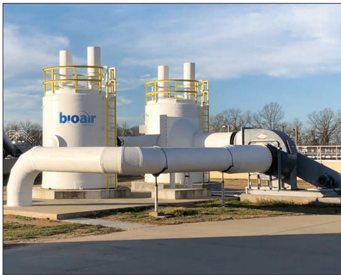
Figure 1. Carbon filter treating 17,000 cubic feet per minute (cfm).
