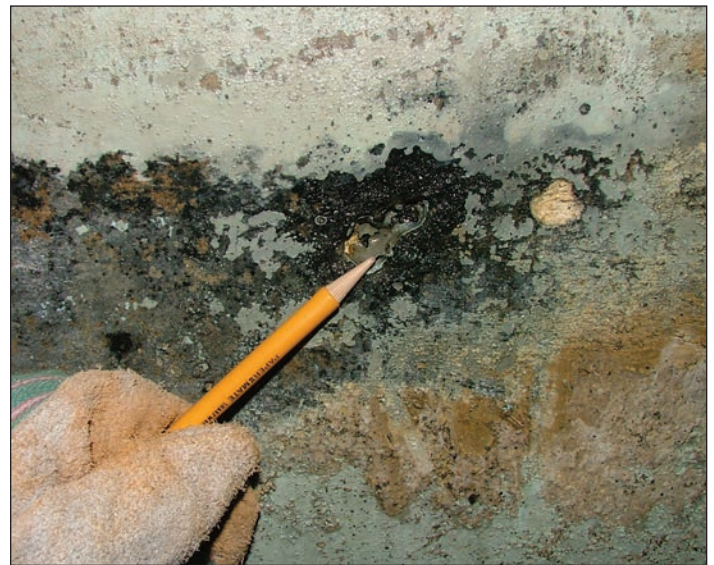
Photograph 2. Primary clarifier headspace with odor control. Deterioration of coatings and concrete after six months of service exposure.
