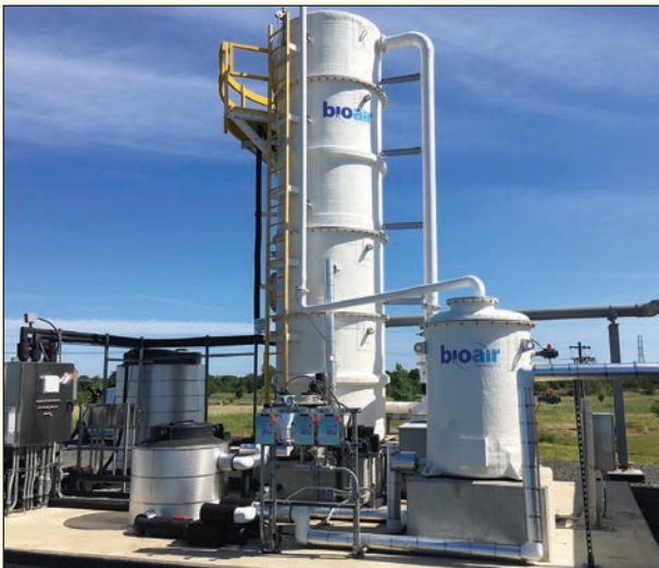
Biotrickling filter for VOC treatment, Superfund site, Bridgewater Township, New Jersey. Rob Firestone
