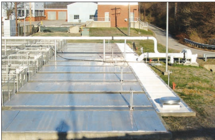
Flat covers over primary clarifier effluent channels. Bowker & Associates
