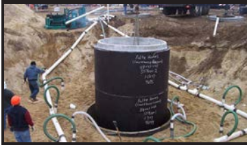
Courthouse Commons Pump Station
