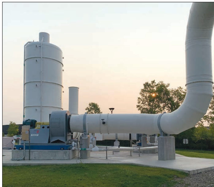
Figure 4. Biotrickling filter treating 25,000 cfm. Rob Firestone
