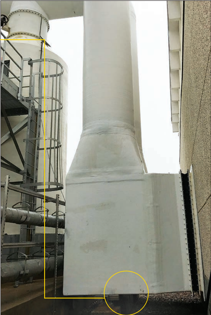
Photograph 3. A repaired vertical scrubber duct section that was improperly supported, cracked and leaked hazardous corrosive condensate.
