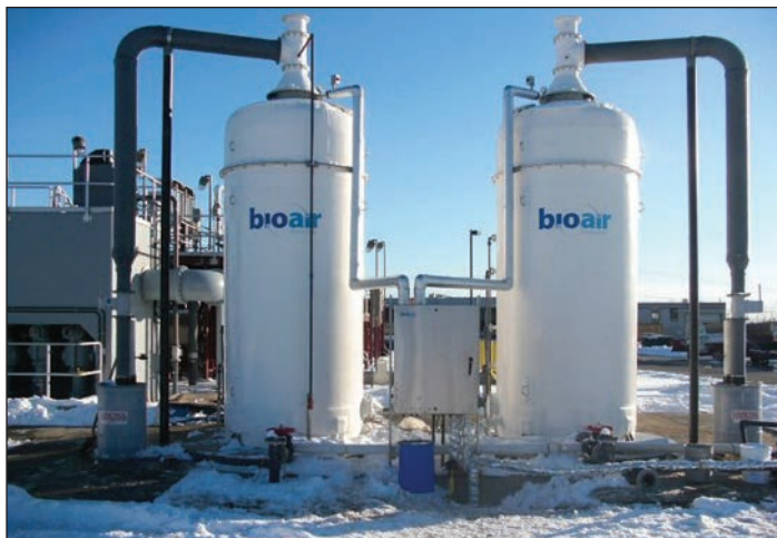
Bioscrubber odor control system.
