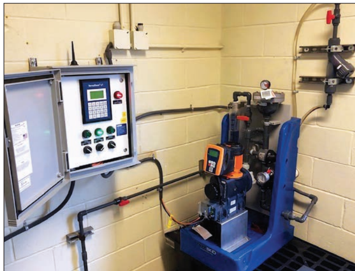
Figure 2. Village of Wolcott advanced dosing controller. Todd Gaignat
