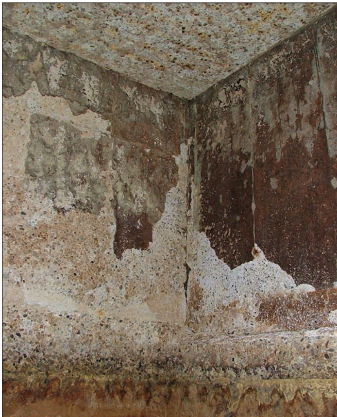
Photograph 5. Grit tank headspace with advanced corrosion with non-operational odor control system. Randy Nixon
