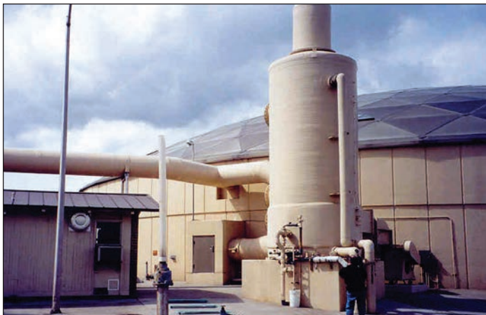
Traditional dome and wet scrubber system.
