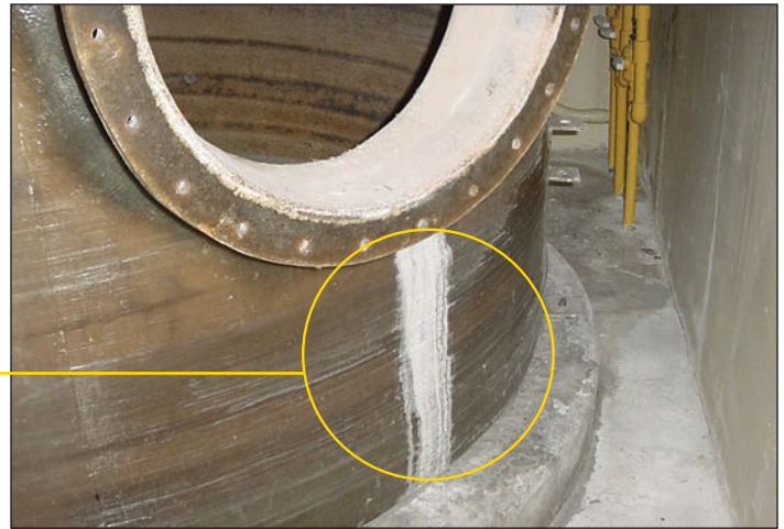
Photo 6. Close-up of FRP deterioration on one of the sodium hypochlorite tanks.
