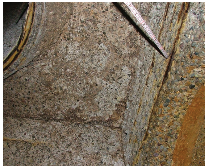
Photograph 3. Pump station wet well headspace with the beginning exposure of rebar with operable odor control.
