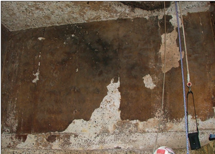
Photograph 4. Pump station wet well headspace with visible surface corrosion with operable odor control. Randy Nixon
