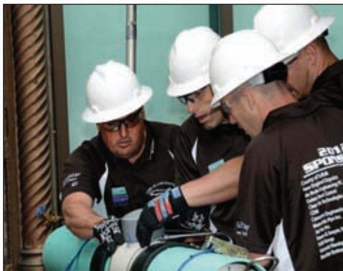
Brown Tide team members work in concert to perform a pipe repair at the Operations Challenge.
