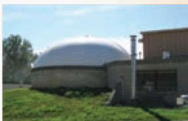
Digester Gas Holding Cover
