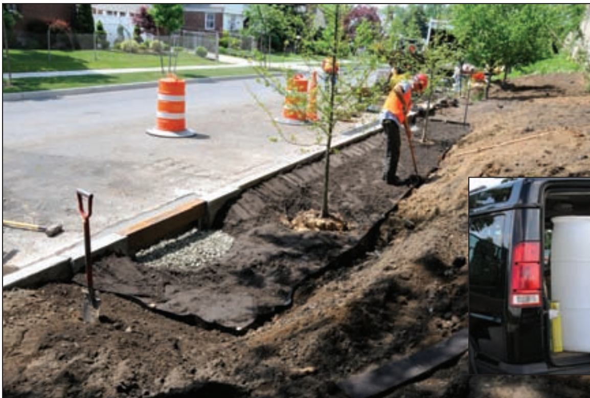
The construction of numerous bioswales and the institution of a rain barrel give-away program are part of the citywide green stormwater management effort.
