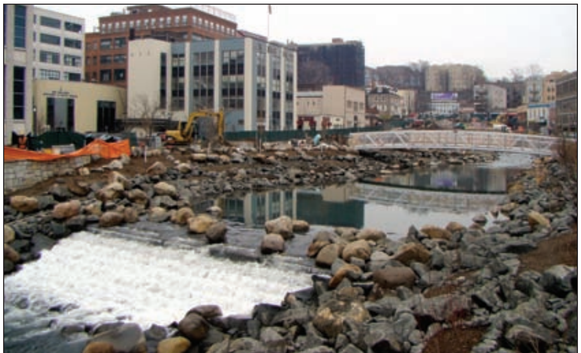
The Sawmill River was daylighted (unearthed) and the hardscaping phase of this GIGP project in Yonkers, NY is shown as it moves forward, nearing landscaping completion this summer. A fish ladder is seen in foreground.
