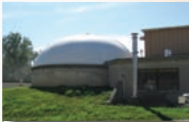
Digester Gas Holding Cover
