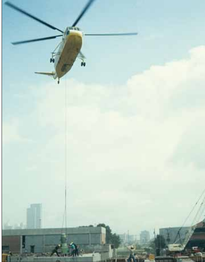
A helicopter lowers the Aeration Mechanical Mixer into place during South Plant construction, during the summer of 1972.
