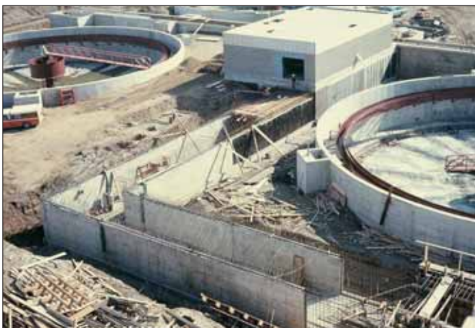
Construction of the North Plant Final Clarifiers and Return Activated Sludge Pump Building, during the summer of 1972.
