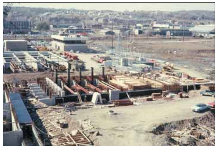
Construction of the North Plant Headworks, Primary Clarifiers and Administration Building, during the summer of 1972.
