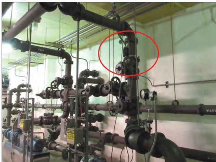
Unit 1 (circled in red) on TWAS pump discharge line
