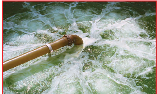
MIXING AND AERATION IN pH CONTROL TANK
