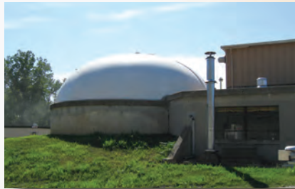
Digester Gas Holding Cover
