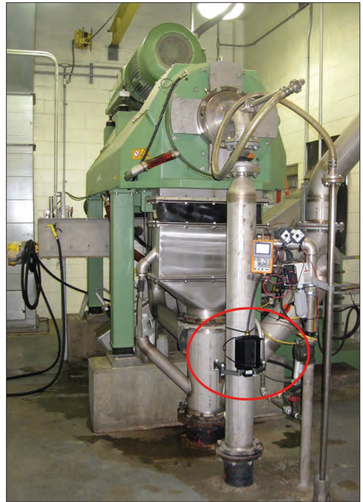
Unit 2 (circled in red) on centrifuge feed piping
