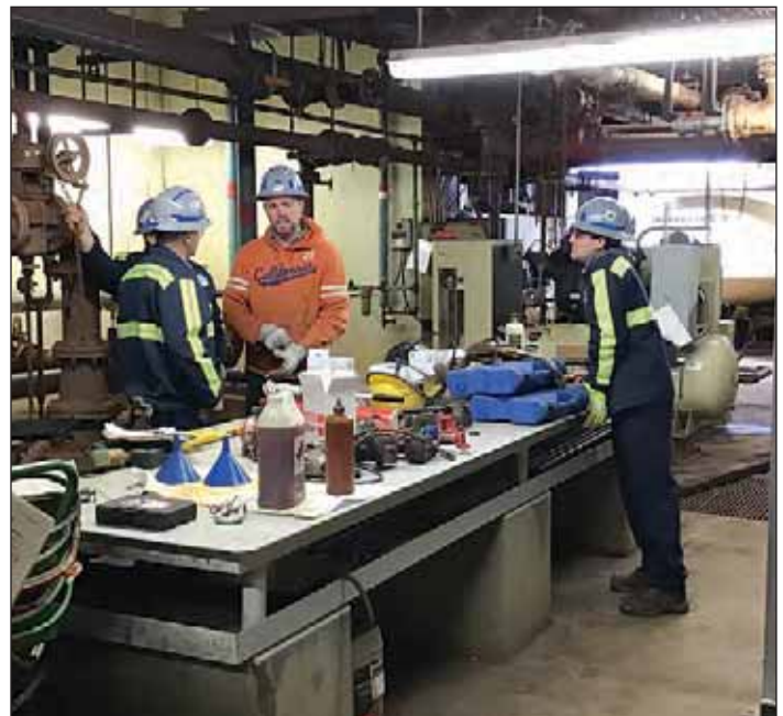
Trainees learning to install new pumps. Pictured from left to right: Todd Nottell, Jay Slate, Chad Putnam and Chris McMahon. R. Mark Crandall
