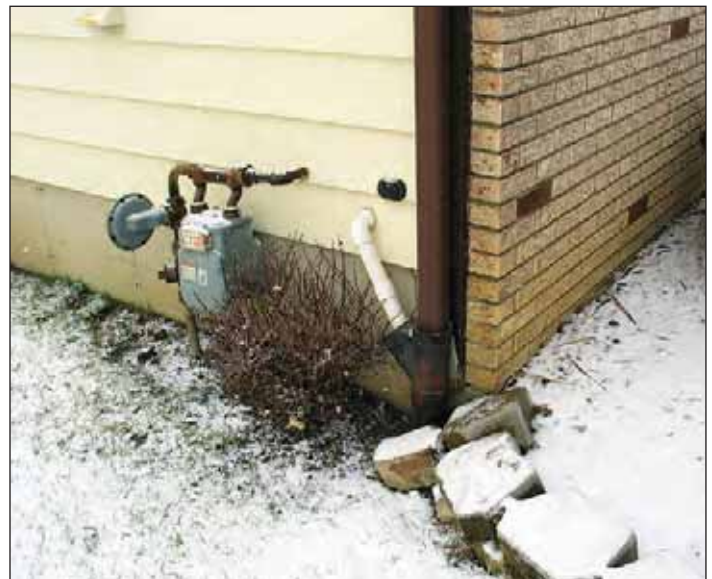
Sump pump and downspout connections below grade may be connected to the sanitary sewer system and should be dye tested to verify where they discharge, as improper connections can expose the property owner to the risk of sewage backup into the home.
