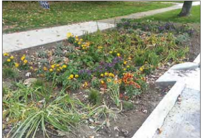
A bioretention cell, or rain garden, installed as part of Buffalo Sewer's CSO 060 Green Infrastructure Project. Buffalo Sewer Authority
