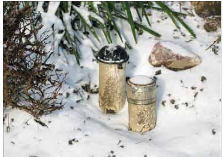
Proper caps for the vent and cleanout reduce the potential for I&I.
