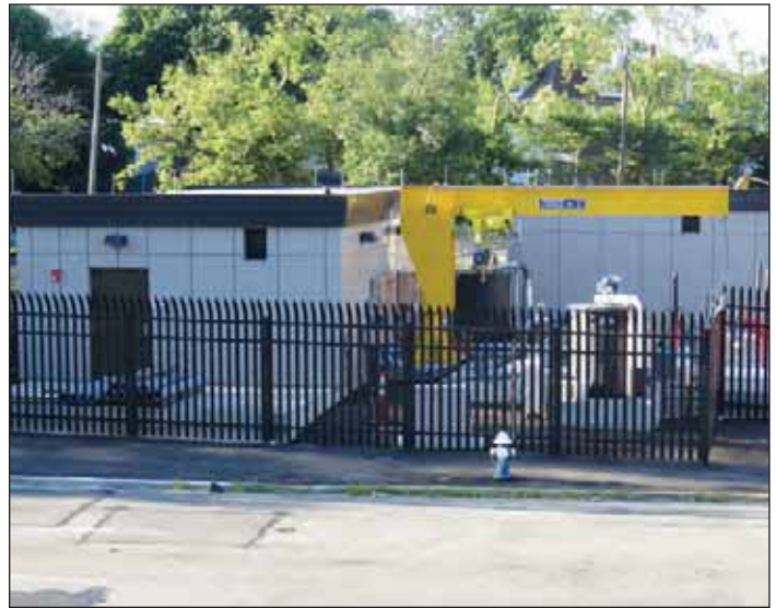
Photograph 5. Pumping Station building and pump hoist, with security fence. Steven Hearl, H2M
