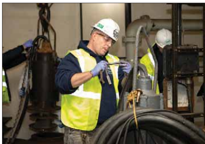
Photograph 3. Collections Sewage Treatment Worker maintaining a main sewage pump.
