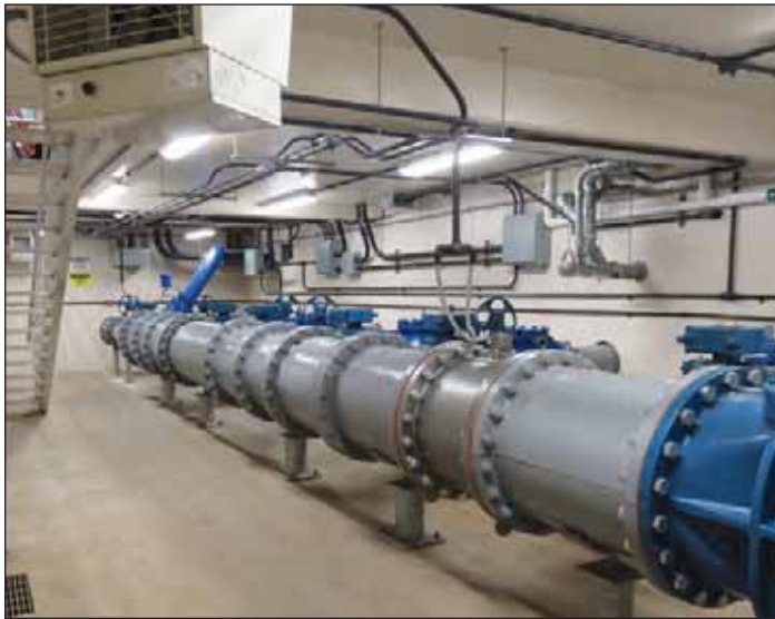
Photograph 3. Valve chamber located on the lower level of one of the buildings of the new pump station. Steven Hearl, H2M
