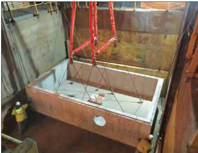
Photograph 4. Placement of the first precast wet well base section. Steven Hearl, H2M
