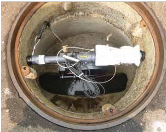
Photograph 2 (top and bottom). Fully stabilized monitors enable high-quality data collection. The units are shown mounted above the invert in each instance. ADS Environmental Services
