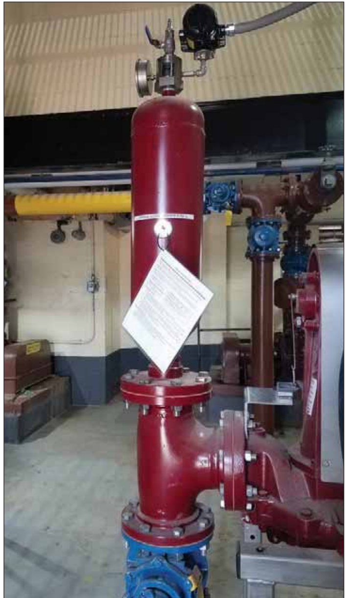
Each piece of equipment has an Energy Control Procedure hanging from it to remind employees about the safety requirements specific to that piece of equipment. The Energy Control Procedure details the hazards involved with the equipment, the safety protocols for de-energizing it for repairs and the process for restoring it back to service. Angel French
