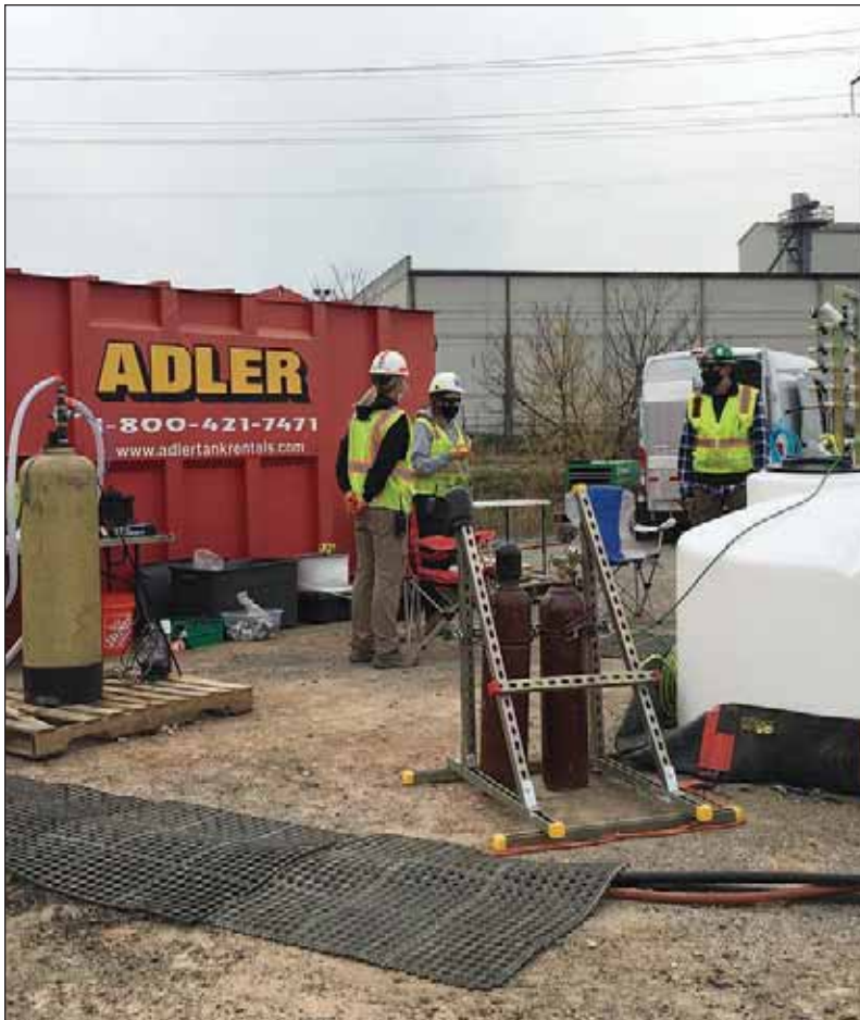
Tripping hazards mitigated and overview of work area as the team practices social distancing and wearing their face masks along with other required PPE.
