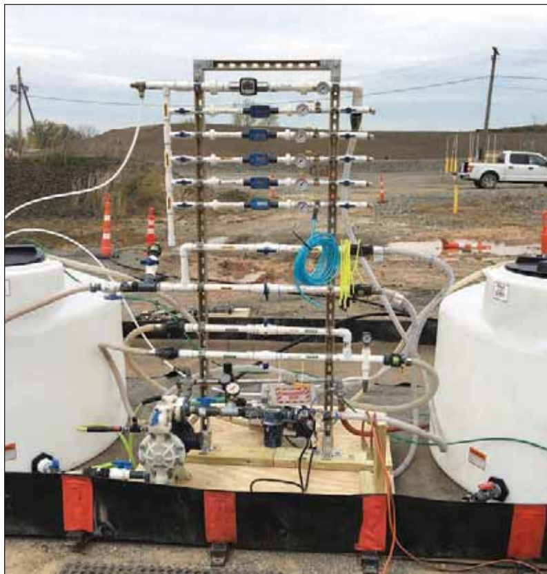
EISB injection manifold and connections to the mixing tanks, which were within secondary containment.
