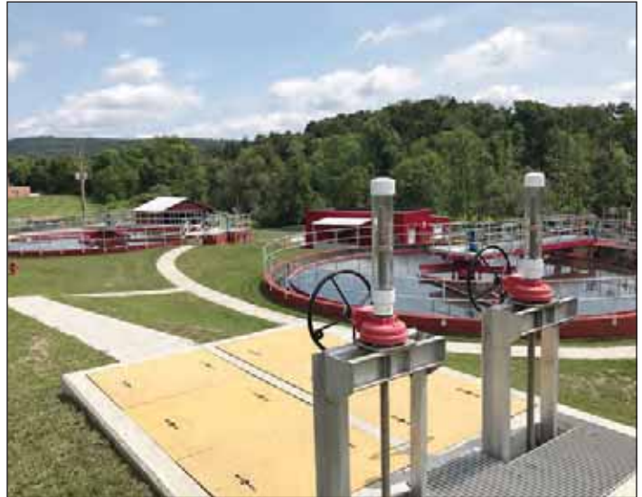
Two new primary clarifiers have been added to the Cooperstown WTP. Jarrett Hotaling
