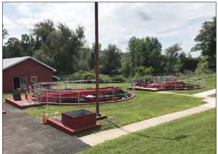
The two existing secondary clarifiers have been outfitted with all new interior components and valving. Jarrett Hotaling
