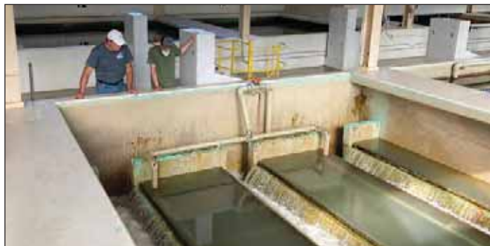
North Tonawanda Treatment plant Water Operator David Conti, left, and intern Elijah Kunze are backwashing a filter.
