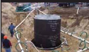
Courthouse Commons Pump Station
