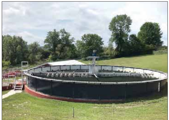
The hydraulically driven trickling filter with rock media has been replaced with a motor-driven distribution assembly and synthetic media. Jarrett Hotaling
