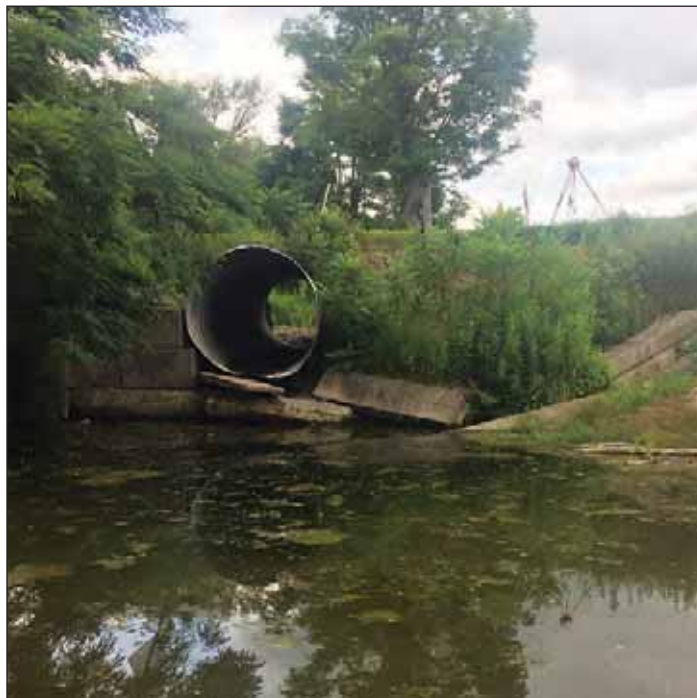
BEFORE: View of the culvert outlet, looking upstream. A 2.1-foot drop-off at the end of culvert effectively prevented aquatic organisms from using habitats upstream.
