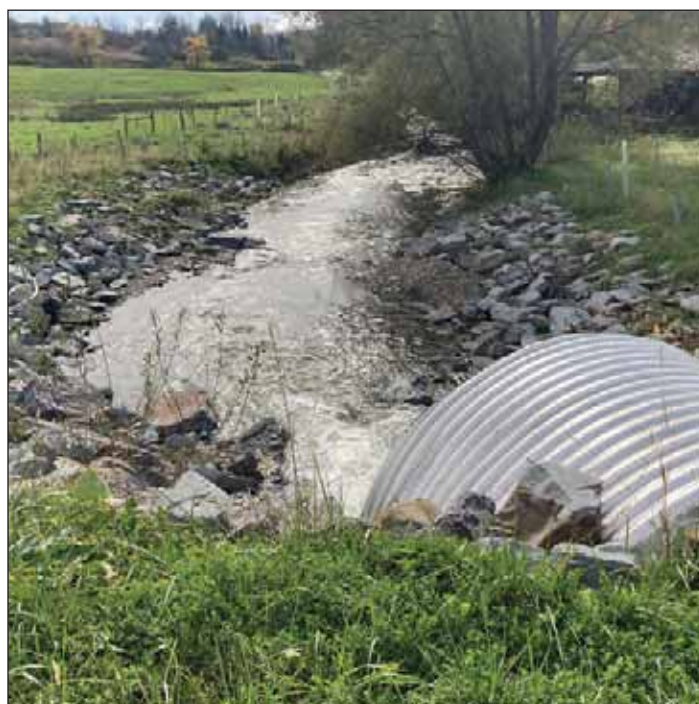
AFTER: View from the culvert outlet, looking downstream. Riprap has stabilized the shoreline, a riparian zone has been planted, and barriers are in place to prevent cows from entering the stream.
