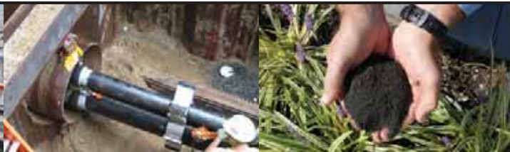
Ronkonkoma Hub Pump Station
