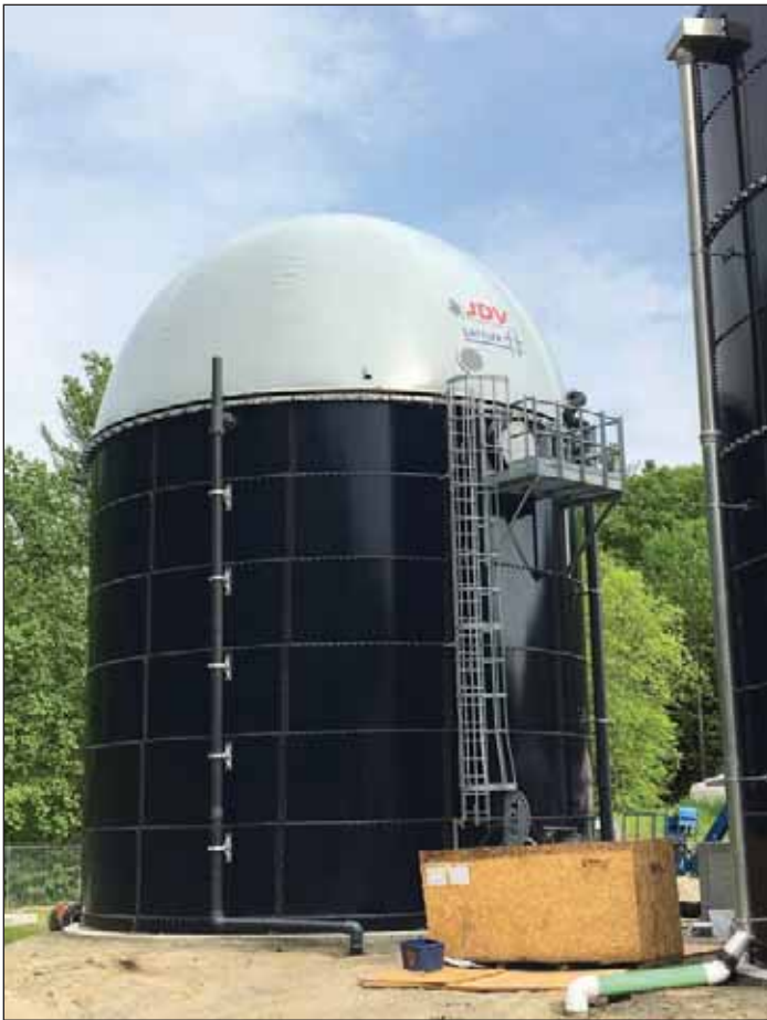
Gas holder, Niskayuna WWTP.
