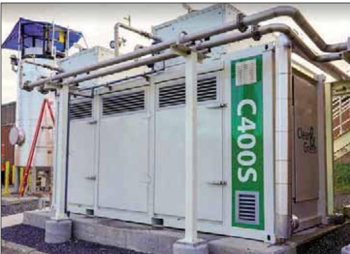
Rome's 400-kilowatt biogas-fired microturbine combined CHP system. George Bevington, Barton and Loguidice
