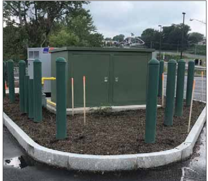
Photo 2. Stormwater pumping station to evacuate stormwater on Culver Road and adjacent parking areas.
