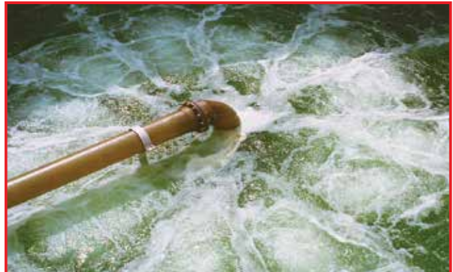
MIXING AND AERATION IN pH CONTROL TANK
