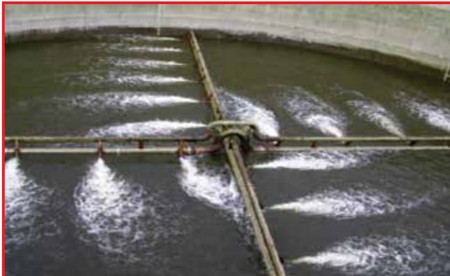
JET MIXING IN EQUALIZATION TANKS
