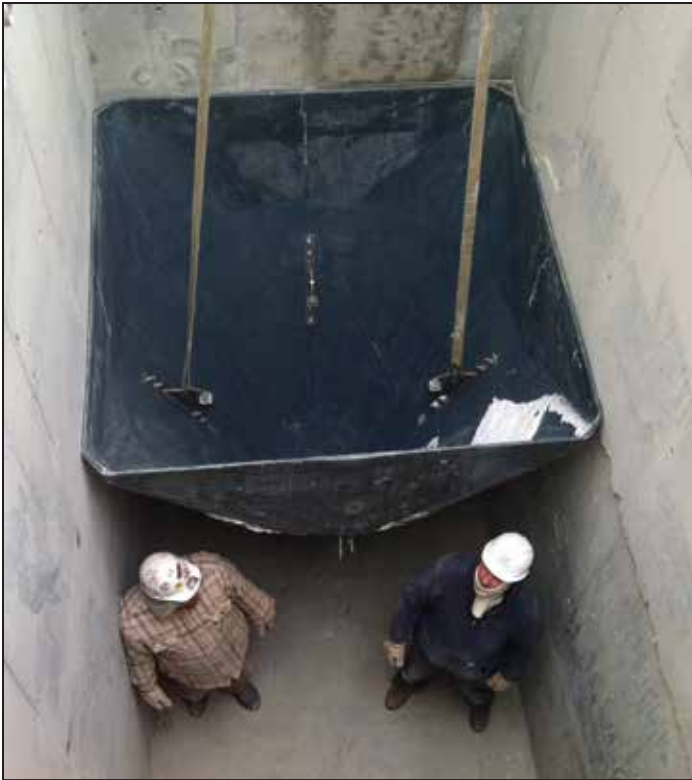
Workers prepare for the installation of the first filter component. The shape of the FRP cone enhances the movement of the filtered water up through the sand.
