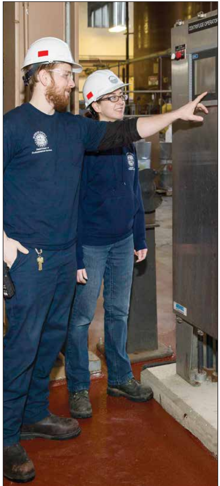
Licensed operators Justin Slentz and Alison Perez, shown reviewing the centrifuge operator panel at the Frank E. VanLare WWTP, a 135 mgd facility operated by Monroe County Department of Environmental Services
