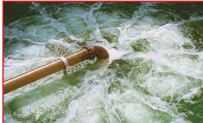
MIXING AND AERATION IN pH CONTROL TANK
