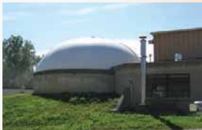
Digester Gas Holding Cover
