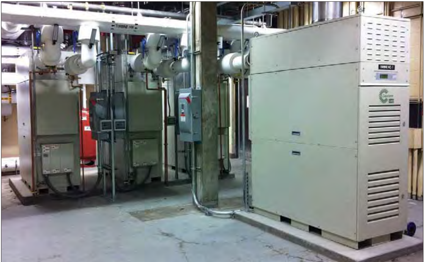
Four 65-kw microturbines for converting biogas into electricity and heat are shown here.
