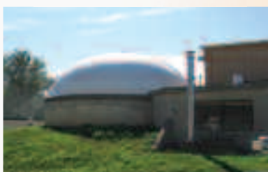
Digester Gas Holding Cover
