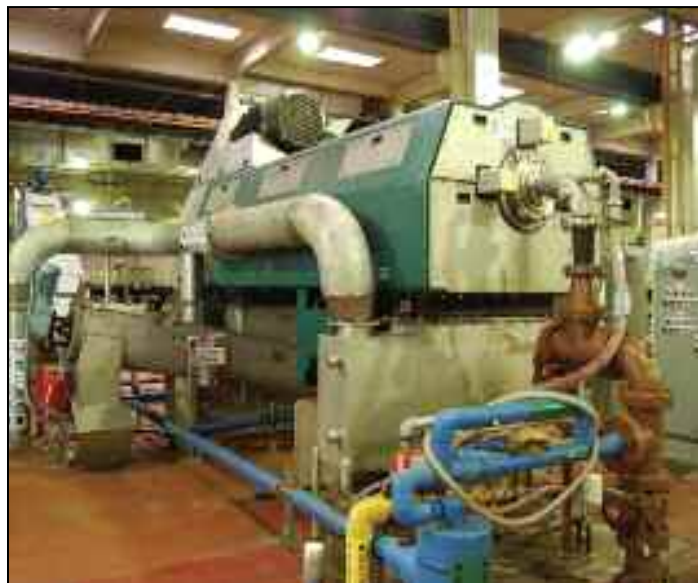
The Buffalo Sewer Authority's dewatering centrifuge removes unwanted wastewater from sludge prior to being conveyed to the incinerator.
