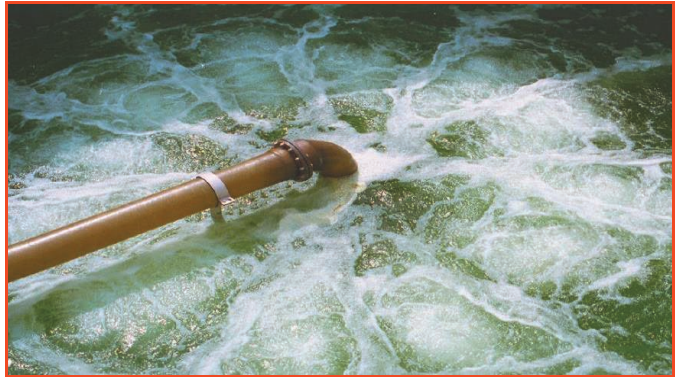
MIXING AND AERATION IN pH CONTROL TANK
