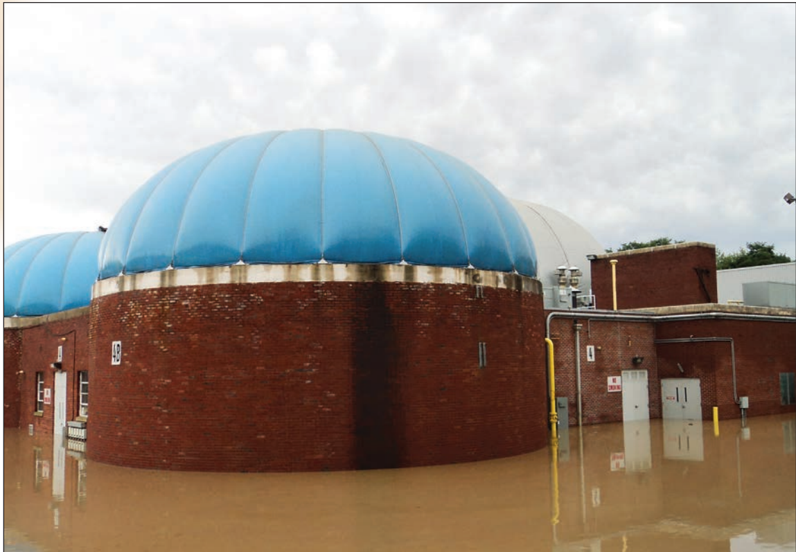
The digesters at the Plant were inundated with floodwaters, before the membrane covers deflated.
