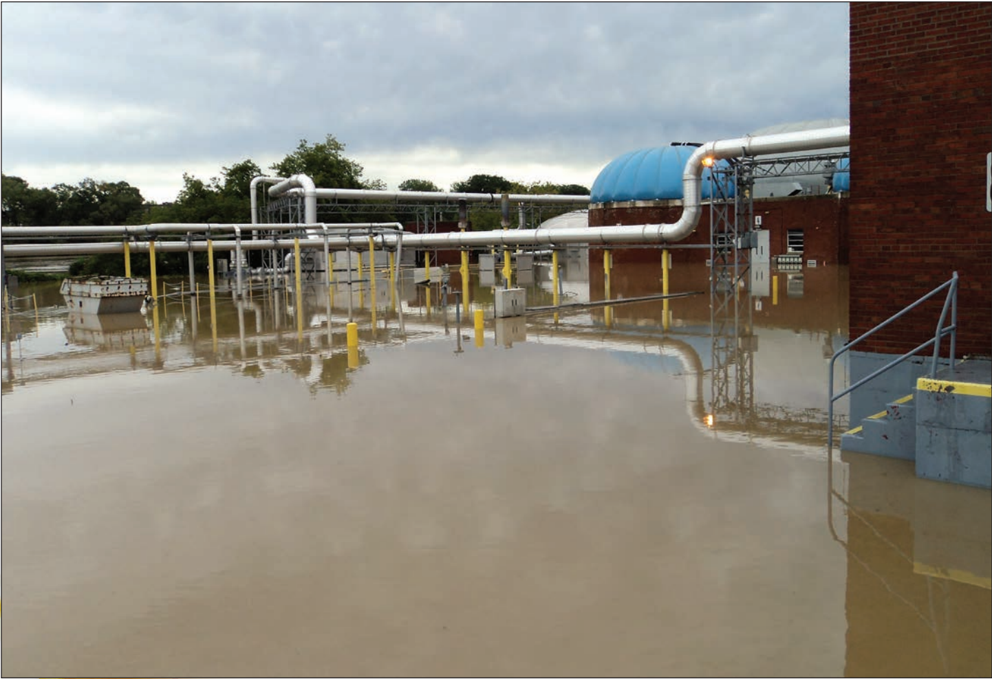
The Plant, looking north over the primary settling tanks, shows them under several feet of water
