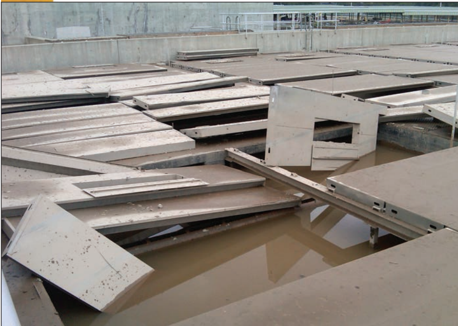
The settling tanks at the Plant were significantly damaged by the flood in September 2011.
