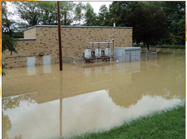
The Terminal Pump Station that services Johnson City and portions of the Towns of Union and Vestal were under record flood waters.
