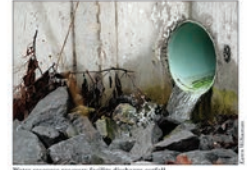
Water resource recovery facility discharge outlet
