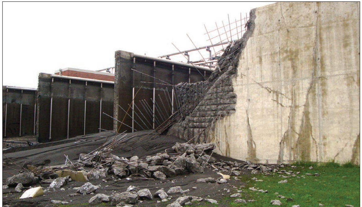
The BAF wall at the Plant experienced a catastrophic failure in May 2011.
