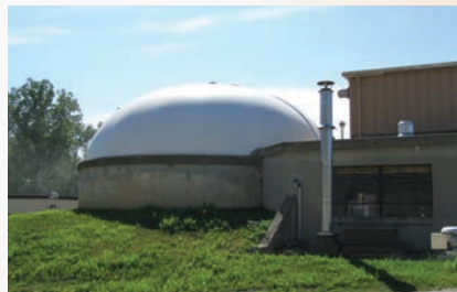
Digester Gas Holding Cover
