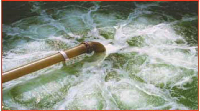
MIXING AND AERATION IN pH CONTROL TANK
