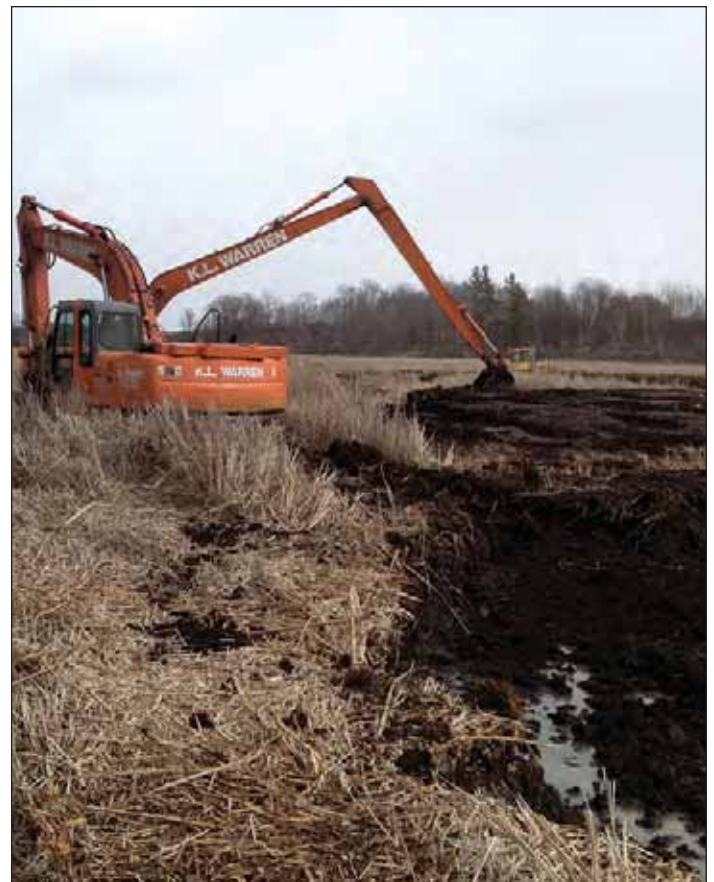
Figure 2. Long-arm excavator works off mats to create potholes and channels to enhance connectivity in wetlands impacted by invasive species.
