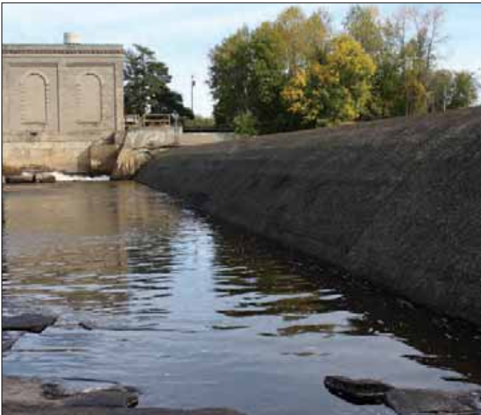
The dam spillway and powerhouse during drawdown. Water is visible flowing through the gates near the powerhouse. Tony David, SRMT
