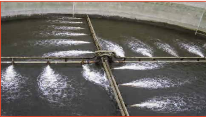
JET MIXING IN EQUALIZATION TANKS
