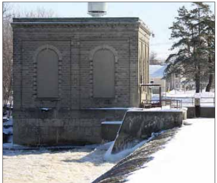
The Hogansburg concrete dam with the pre-cast, concrete-block powerhouse as it appeared in March 2011. Ice cover is visible on the impoundment side of the dam.
