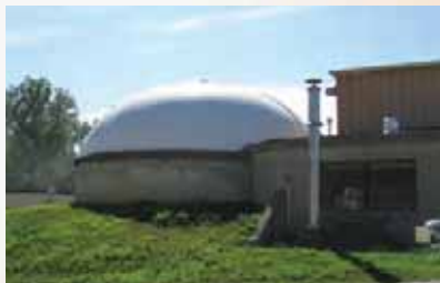
Digester Gas Holding Cover
