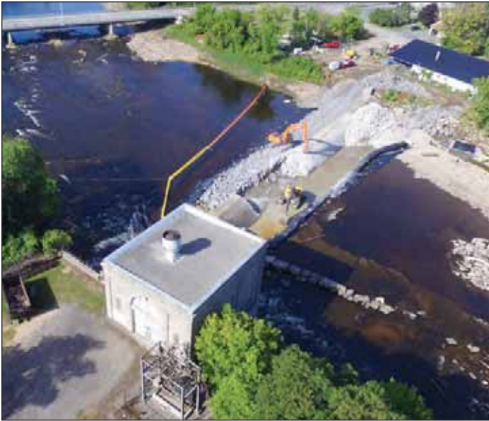
During the demolition phase of dam removal, a coffer dam placed upstream redirected flow around the work area. Kingsburg Companies, LLC
