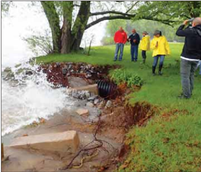
Shoreline erosion inspections along Lake Ontario during the 2017 high water event. U.S. Army Corps of Engineers
