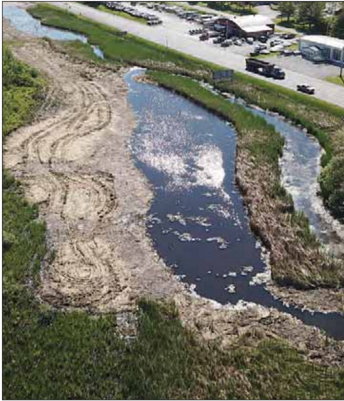
The Otter Creek Restoration Project involves digging up cattails to create potholes, which attract waterfowl and facilitate biodiversity.
