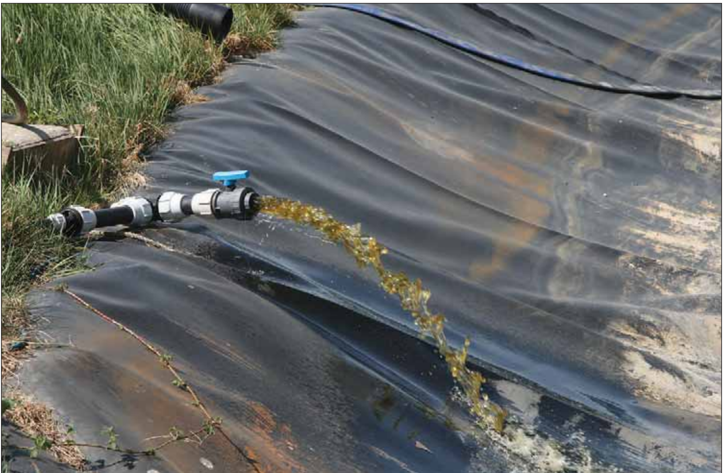
Leachate collected from below the landfill is pumped into a holding lagoon.
