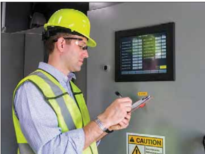
Photograph 5. An operator monitors control room operations in the Varick CORE recycling facility.
