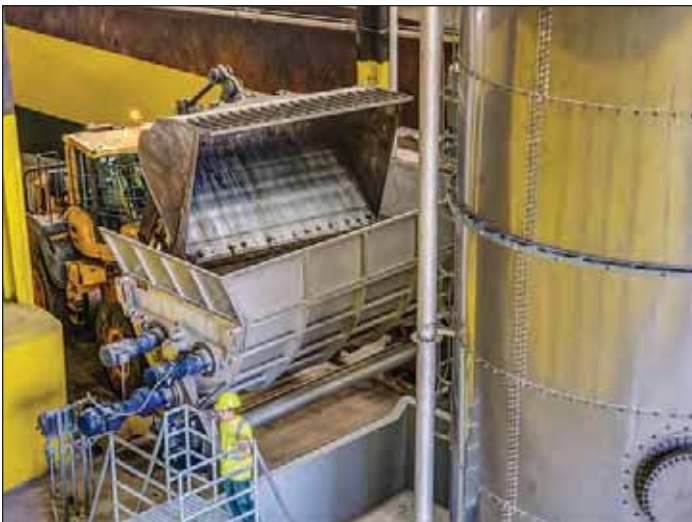
Photograph 4. The Varick CORE recycling facility houses the processing equipment that produces the EBS for the demonstration project.
