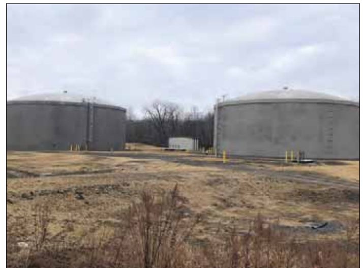
Photograph 5. The new deicing fluid storage tanks at the airport were completed in 2019. Credit: OCDWEP
