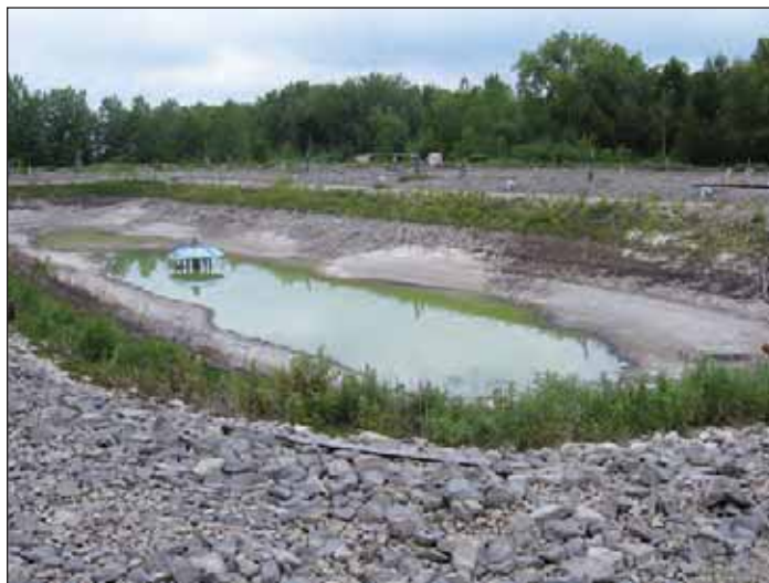
Photograph 4. The treatment lagoons were drained before construction of the deicing fluid storage tanks. Credit: OCDWEP
