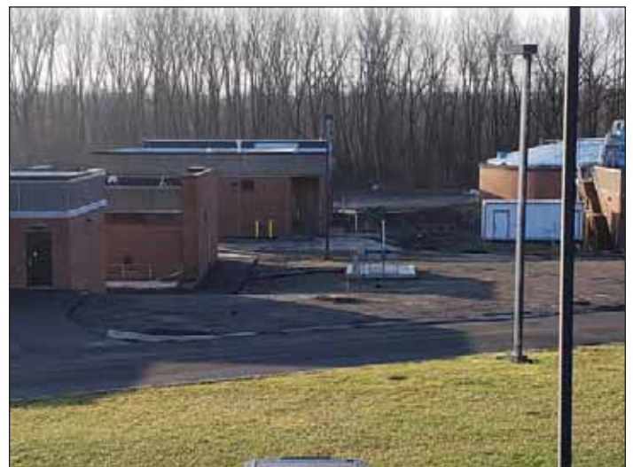
Photograph 2. Newly constructed UV Building (front left) and upgraded Solids Handling Building (back left). Credit: Richard Kenealy
