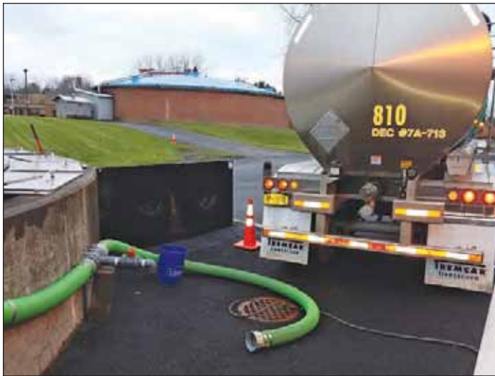
Photograph 4. Thickener tank retrofitted to a high strength receiving station. Credit: Richard Kenealy
