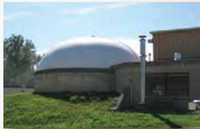
Digester Gas Holding Cover
