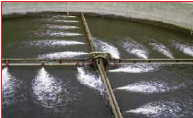
JET MIXING IN EQUALIZATION TANKS
