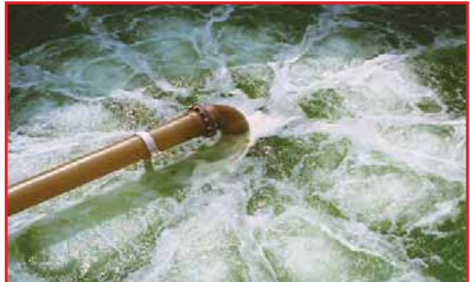
MIXING AND AERATION IN pH CONTROL TANK
