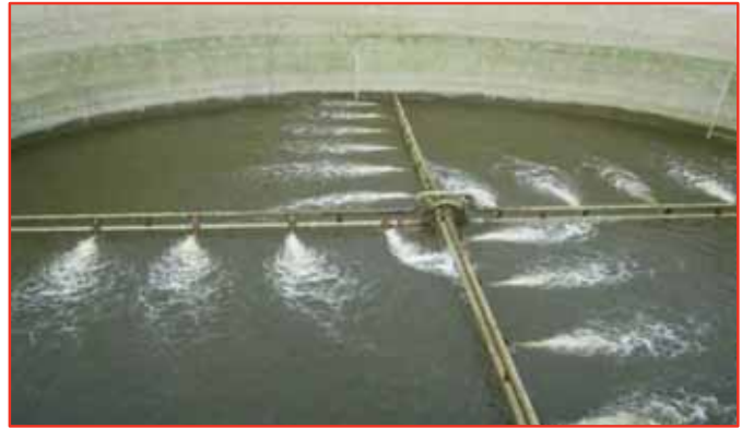
JET MIXING IN EQUALIZATION TANK
