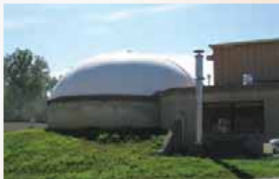
Digester Gas Holding Cover
