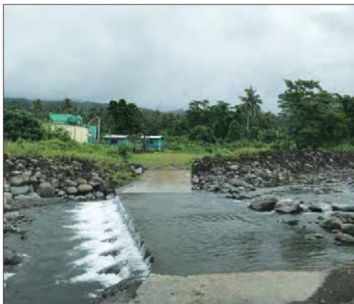
Tasitolala Drinking Water Facility, Samoa Water Authority. The 2012 Tropical Cyclone Evan changed the path of the facility's water source, requiring a reconstruction of the plant's intake and modifications to equipment. NYCDEP
