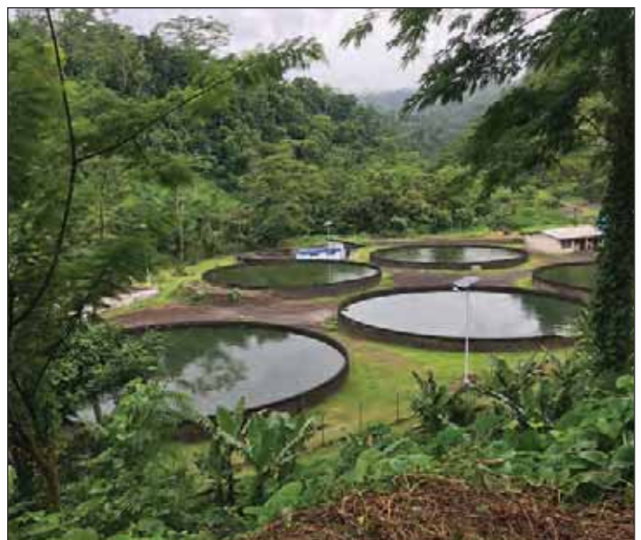
Alcoa Drinking Water Plant, Samoa Water Authority. This facility serves the capital of Apia and shuts down once to twice per month due to site flooding, requiring the use of more expensive alternative water supplies. NYCDEP
