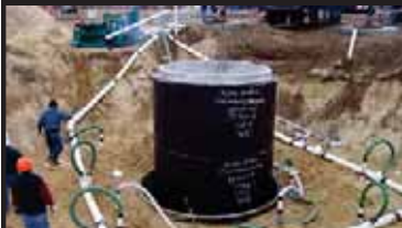
Courthouse Commons Pump Station
