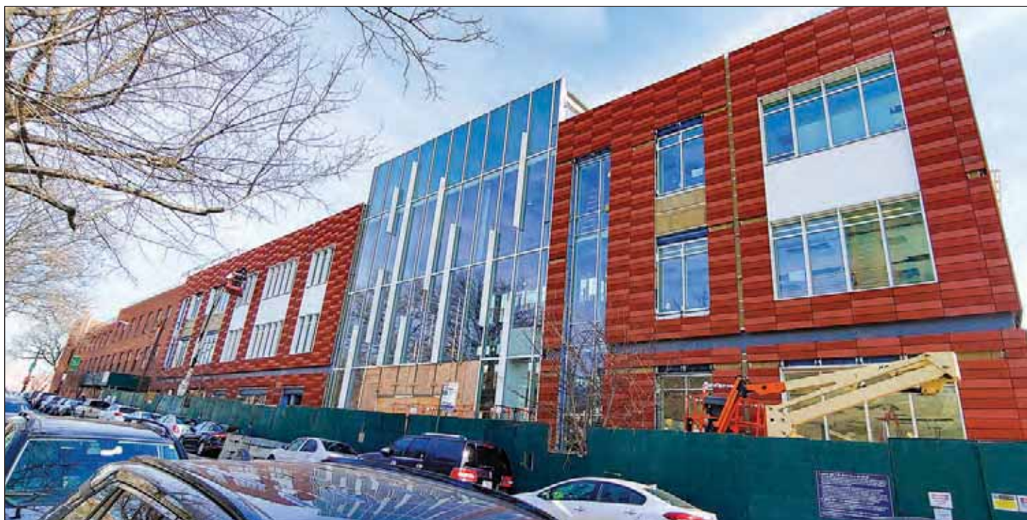
Exterior of the Higgins Engineering and Science Center, under construction in February 2020.
