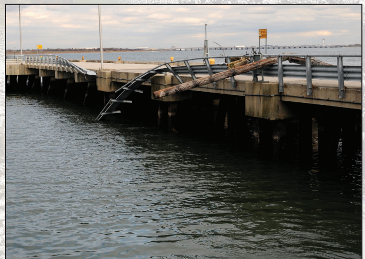
Storm damage at Brooklyn's 26th Ward Wastewater Treatment Plant dock used by sludge vessels
