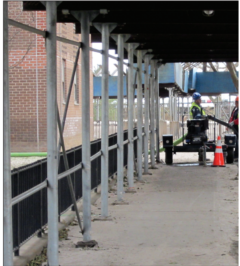
The team had to maneuver pumps into place by hand due to the sand and debris
