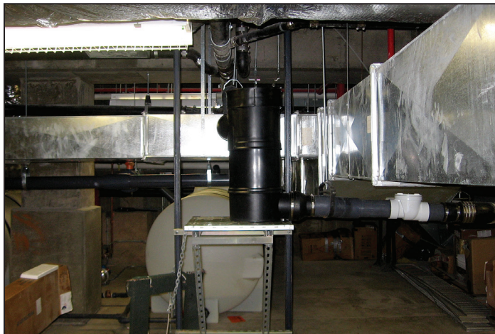
Components of the rainwater collection system included: these white tanks for the rainwater's storage vessels; the rainwater's treatment system in the blue canisters; and the first-flush diverter section (in black).
