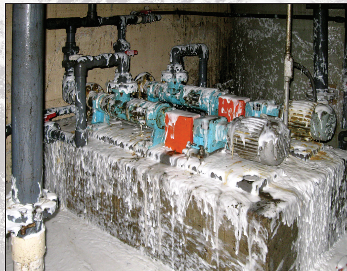
Damage from flooding in the secondary polymer room of the Yonkers treatment plant.
