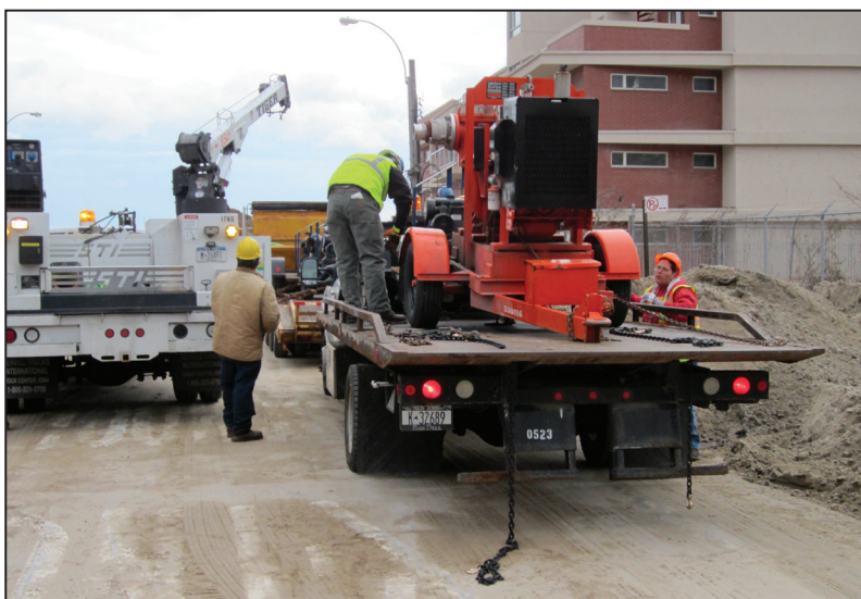
The New York City Housing Authority plowed away sand and debris to make a landing area for the WEP team to begin its work.
