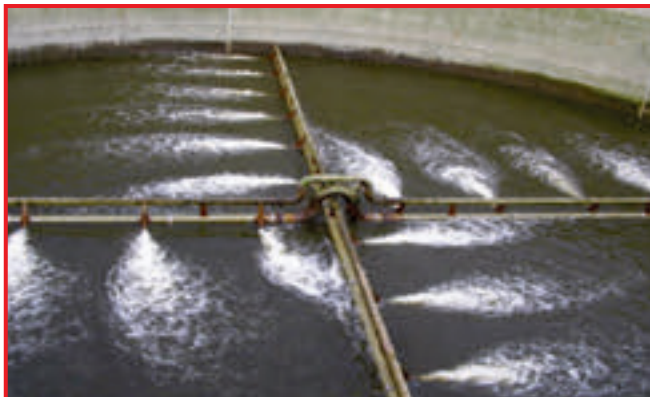
JET MIXING IN EQUALIZATION TANKS
