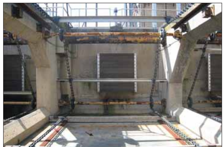
Figure 5. Energy-dissipating baffle, with dimensions of 60 inches by 72 inches, in Tanks 5 through 8. Krish Ramalingam
