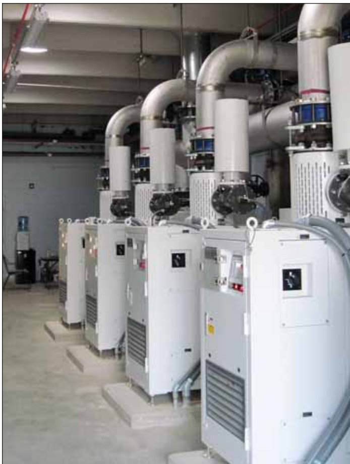
High efficiency blowers have made substantial penetration into the wastewater market over the last 10 years.
