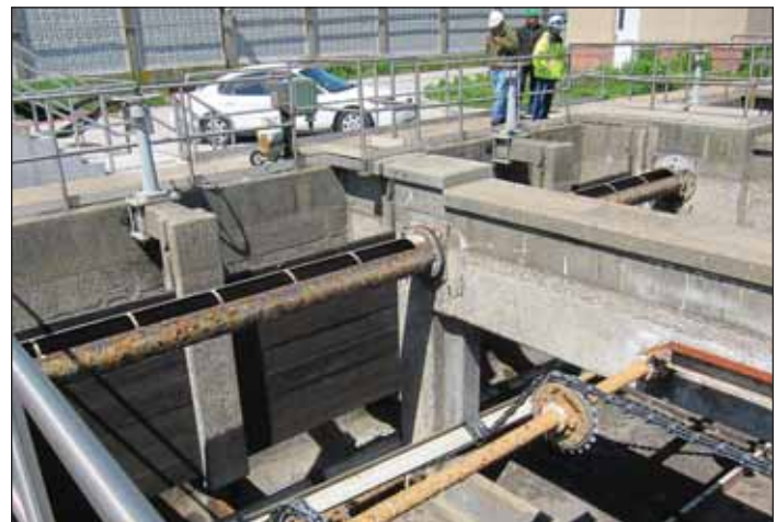
Figure 4. Energy-dissipating baffle along the width, 30-inch opening at the bottom, in Tanks 1 through 4. Krish Ramalingam
