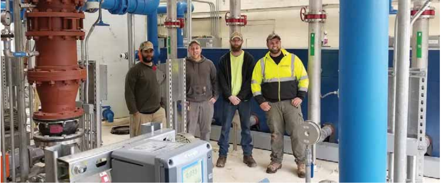
MBR Equipment Room with operators (l-r), Ellie Patton, John Barton, Mike Herbert and Kyle Schmidt.
