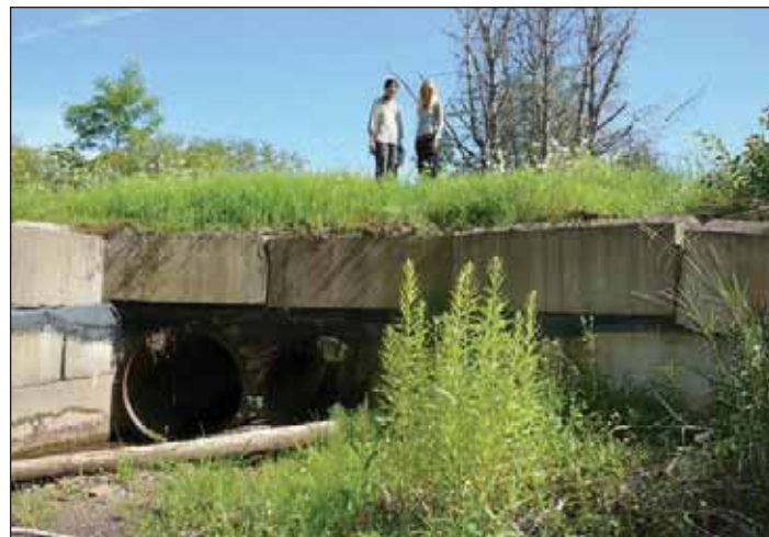
A photograph from 2016 of the old culvert, which had two 36-inch diameter pipes, for a total width of 72 inches. Pictured are Rifat Salim (left) and JoAnne Castagna, Public Affairs. Graydon Dutcher
