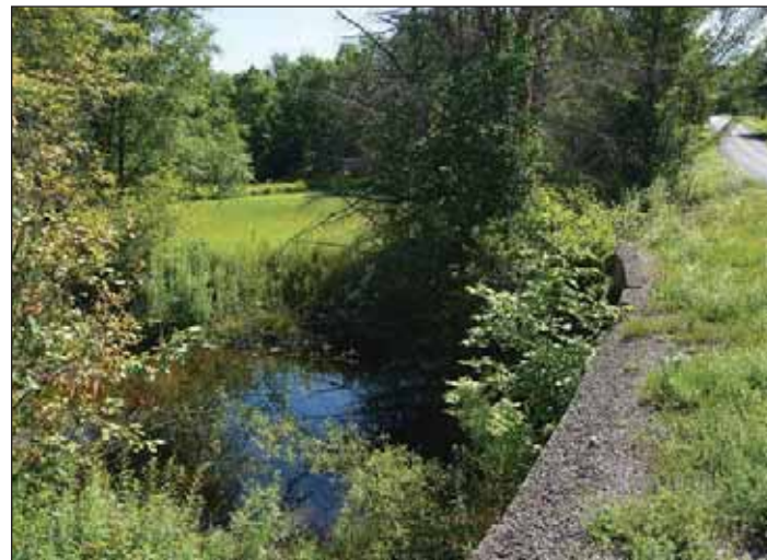
The old culvert's stream banks filled with shrubs and debris in 2016.
