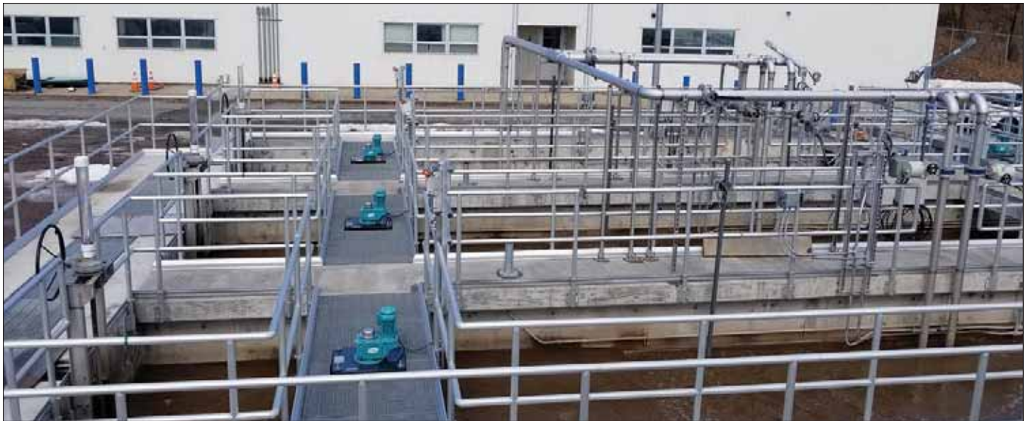
Bioreactors. Aerial view looking at first stage anoxic zones and mixers of BNR system.
