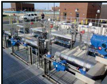
120 MGD UV Disinfection System
