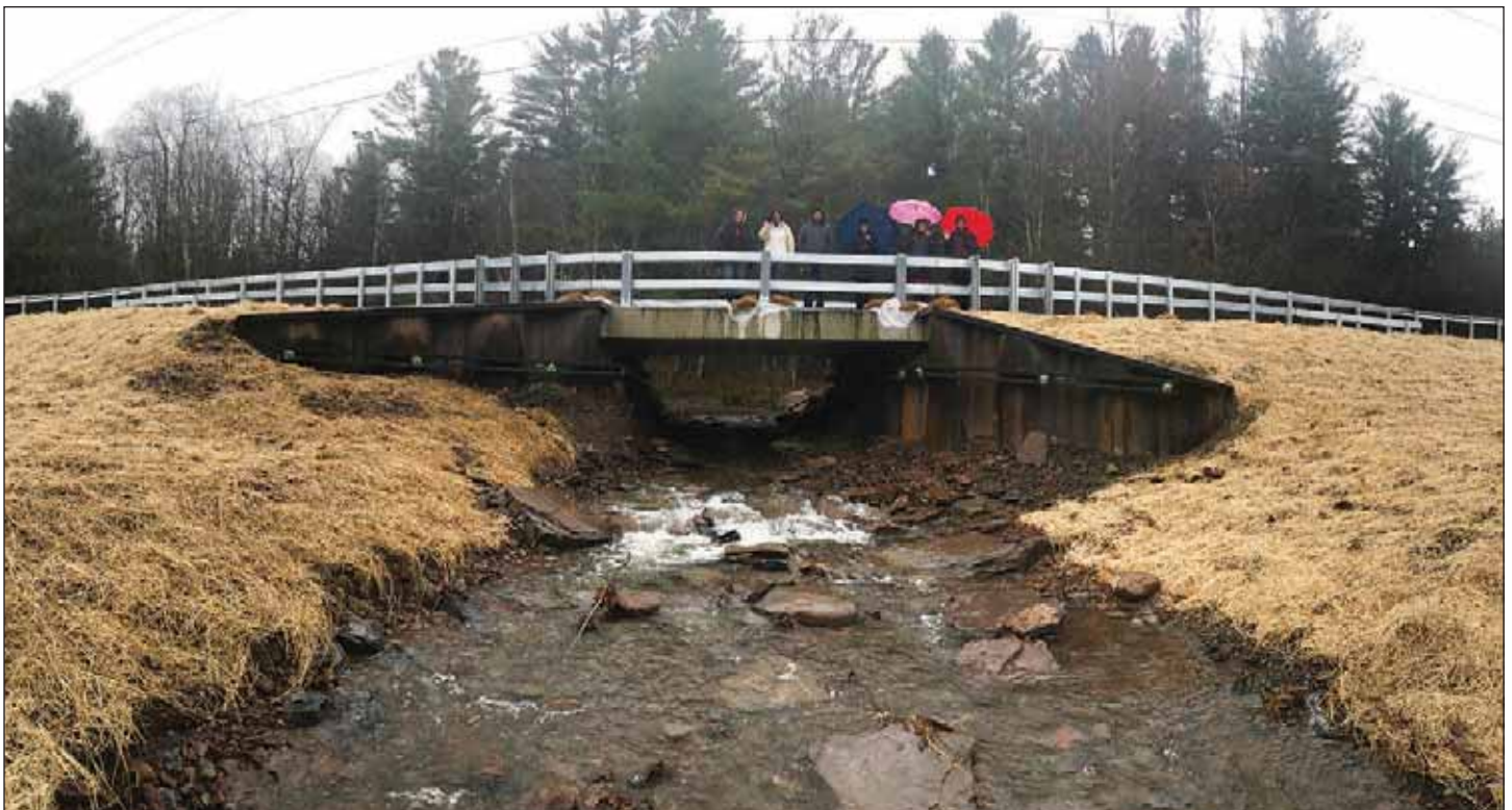
The project team looking over the new culvert as it works successfully in torrential rain conditions in November 2018.
