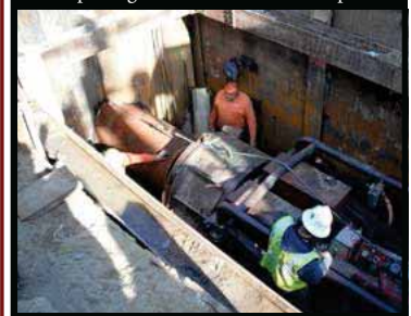
Flow Diversion Project
