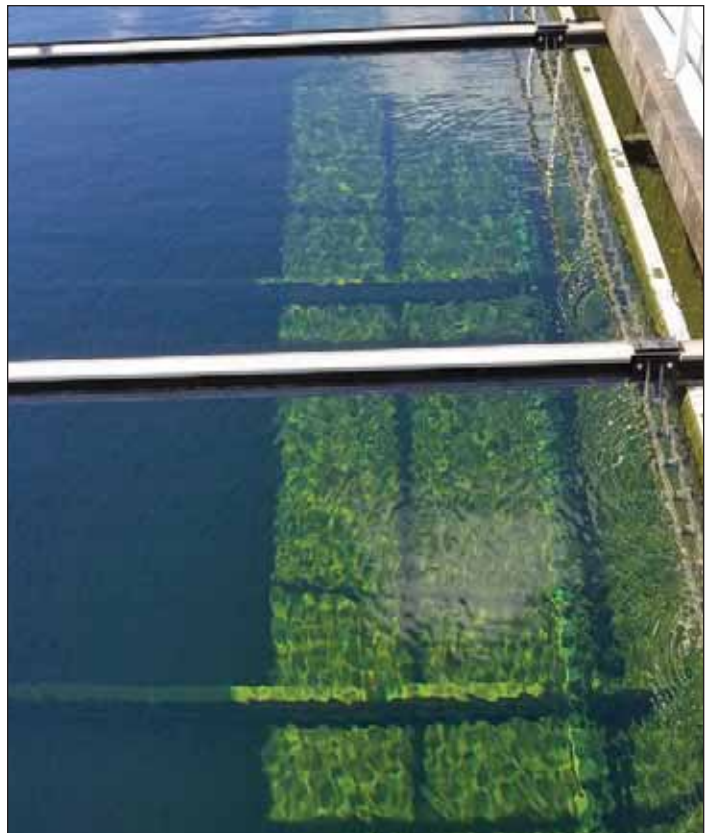
Membrane effluent in FST. MBR effluent flows through the FST influent channel and tanks to prevent freezing of these wet weather tanks in winter. Vincent Apa
