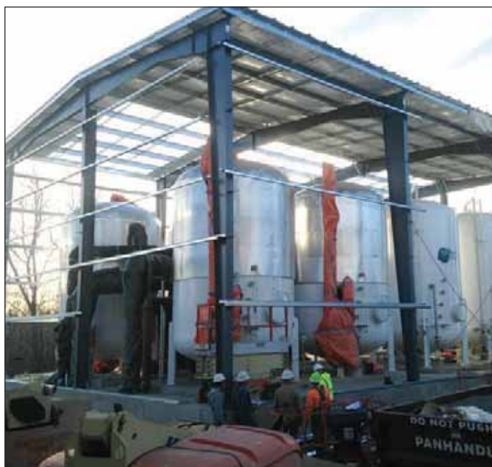
Figure 9. PFAS treatment system.
