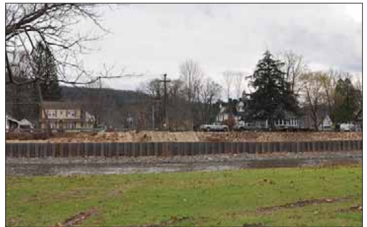
Photograph 5 (after). The West Branch Delaware River and completed South Street Bank Restoration Project in the Town of Walton, as seen from the Walton floodplain.
