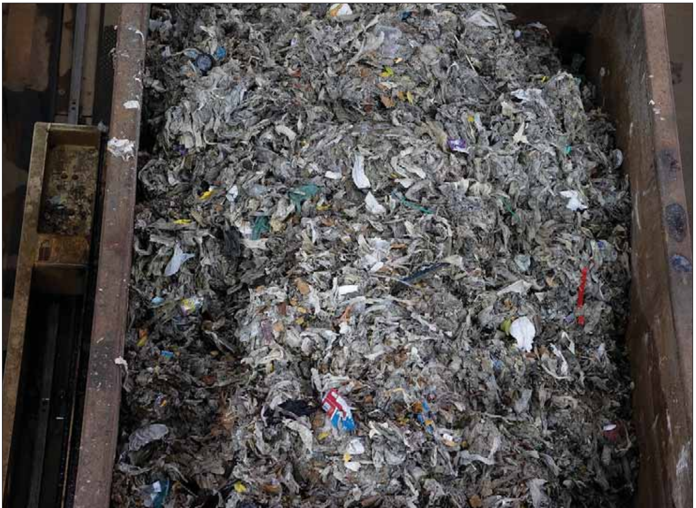
A dumpster full of screenings, overwhelmingly wipes.
