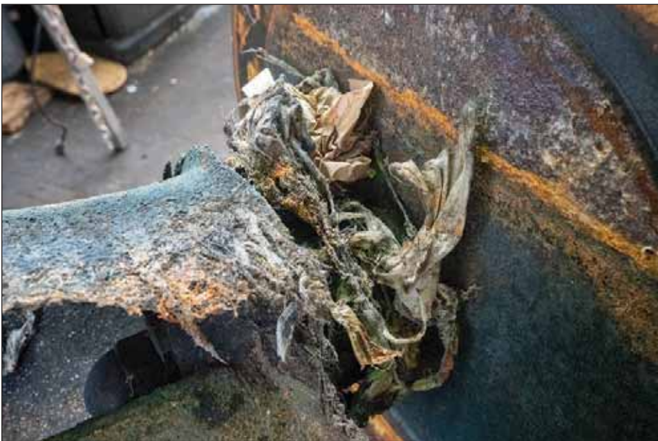
Wipes bound around impeller hub, E Battery RAS pump. Jean Schwarzwald/DEP
