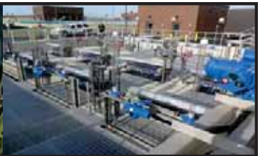
Bergen Point WWTP
