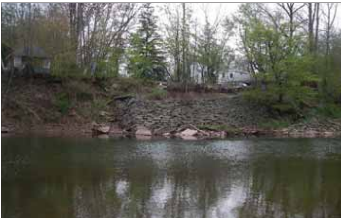
Photograph 3 (before). Stone wall sliding down into the West Branch Delaware River at South Street.
