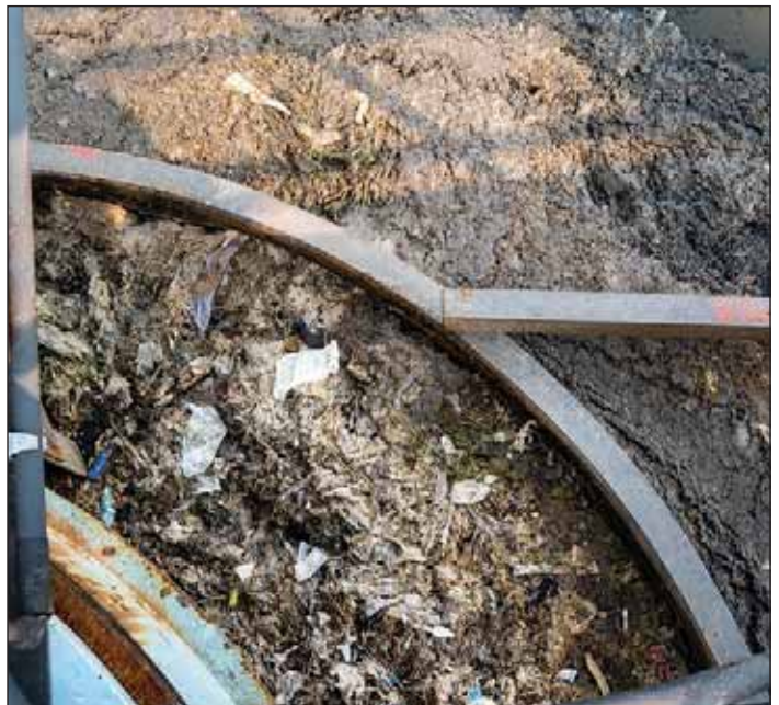
Distribution box of thickener clarifier clogged with rags. Jean Schwarzwald/DEP
