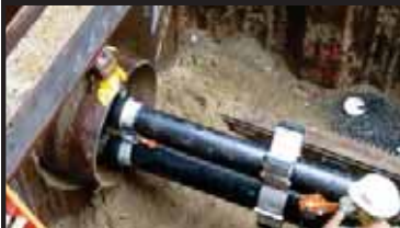
Ronkonkoma Hub Pump Station
