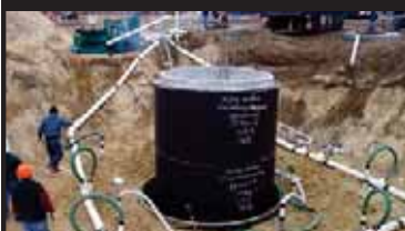
Courthouse Commons Pump Station
