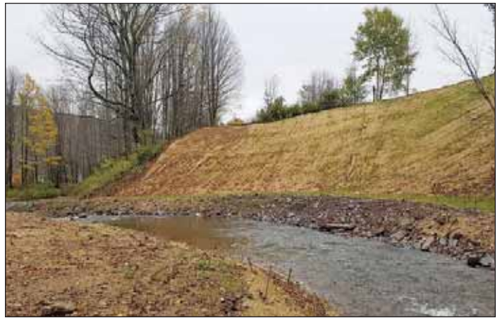
Photograph 8 (after). The completed Hardscrabble Streambank Stabilization Project in the Town of Roxbury in late 2019. JoAnne Castagna
