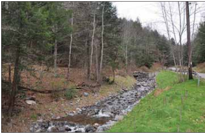
Photograph 7 (after). Completed Close Hollow Streambed and Bank Restoration Project in the Town of Andes in late 2019. JoAnne Castagna
